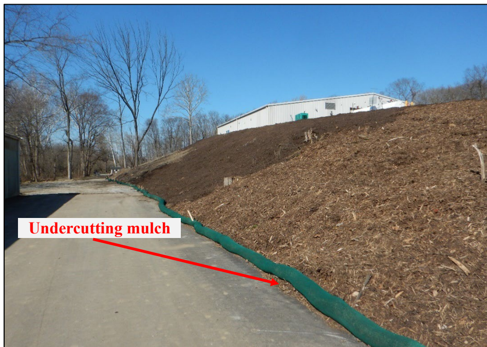
Photograph 44. Township Public Works Campus: (DSCN2938) View, facing north, of the steep slope in between the upper garage and lower garages. The Township had placed mulch on the slope to assist with erosion and had staked filter socks at the toe. However, the mulch was undercutting the filter sock, which was also not staked.
