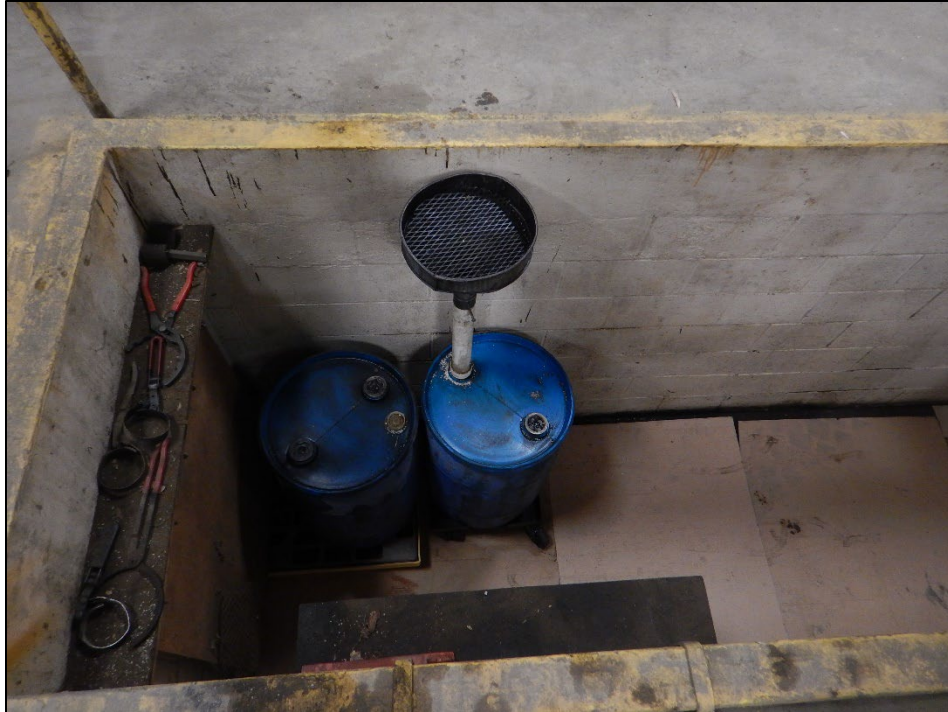
Photograph 38. Township Public Works Campus: (DSCN2922) View, inside the upper garage, of the fluid draining pit that the Public Works staff use for servicing vehicles. There were no drains in the pit.
