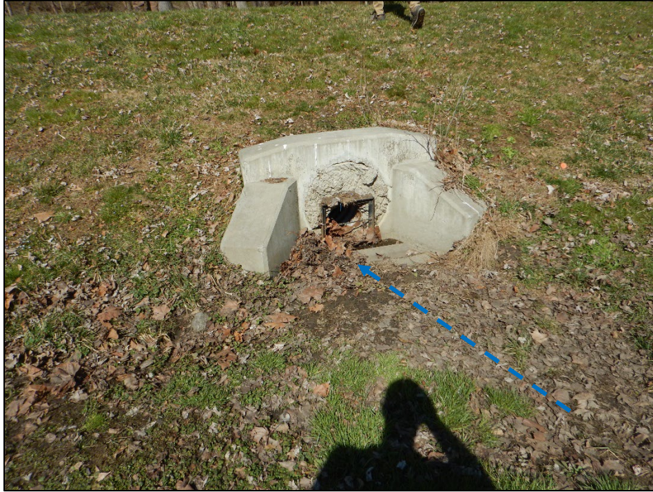
Photograph 19. Chadwick Circle Detention Basin: (DSCN2869) View, facing northwest, of the outflow headwall that conveys stormwater to an adjacent vegetated ravine. Note the blue arrow indicating the direction of flow.
