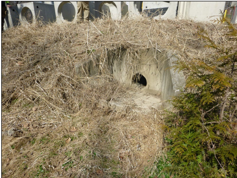
Photograph 42. Township Public Works Campus: (P1060613) View, facing north, of the stormwater headwall and outlet pipe that receives stormwater flow from the adjacent Campus parking lots/roads. Stormwater flows from this outlet pipe into a vegetated area.
