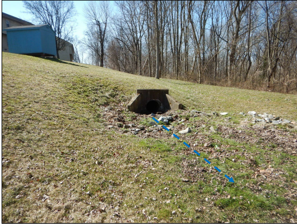
Photograph 21. Chadwick Circle Detention Basin: (DSCN2866) View, facing southwest, of the basin inflow headwall. The riprap in the forebay needed maintenance and replacement. Note the blue arrow indicating the direction of flow.
