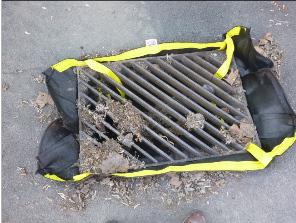
Photograph 43. Township Public Works Campus: (P1010614) View of a drop inlet with filter insert located in the parking area for the Campus. Stormwater conveys through the inlet and out the headwall, as shown in Photograph 42.
