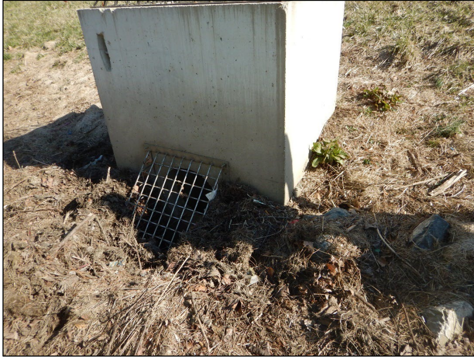
Photograph 11. Kensington Club Basin Rehabilitation Project: (DSCN2848) Closer view of the basin's concrete outlet structure, as shown in Photograph 10. The lowest outlet, behind the visible trash rack, was inundated with sediment and debris.
