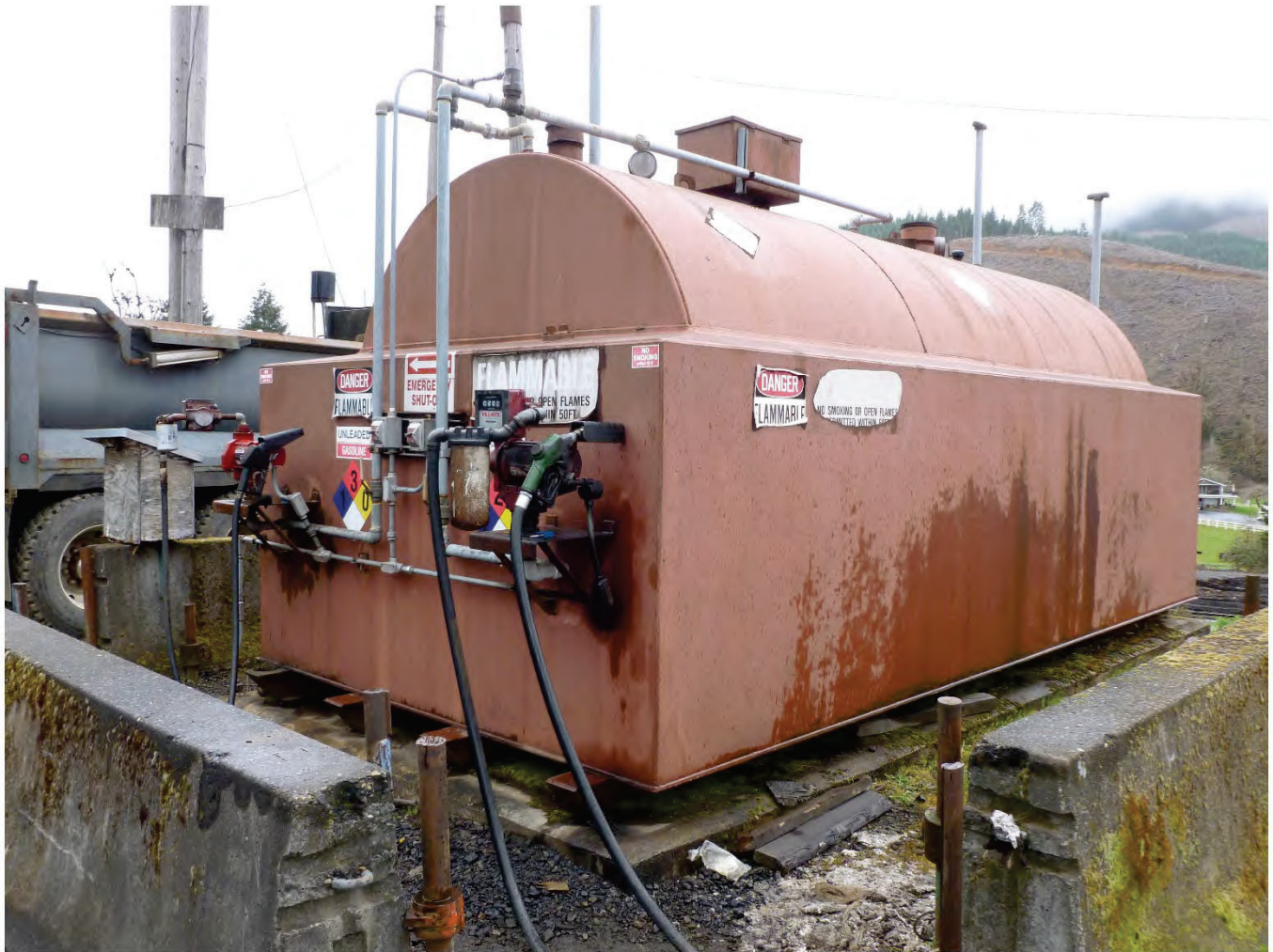
Photo 1 / P1000814 – Gas/Diesel Tank, double-walled, side, facing west
