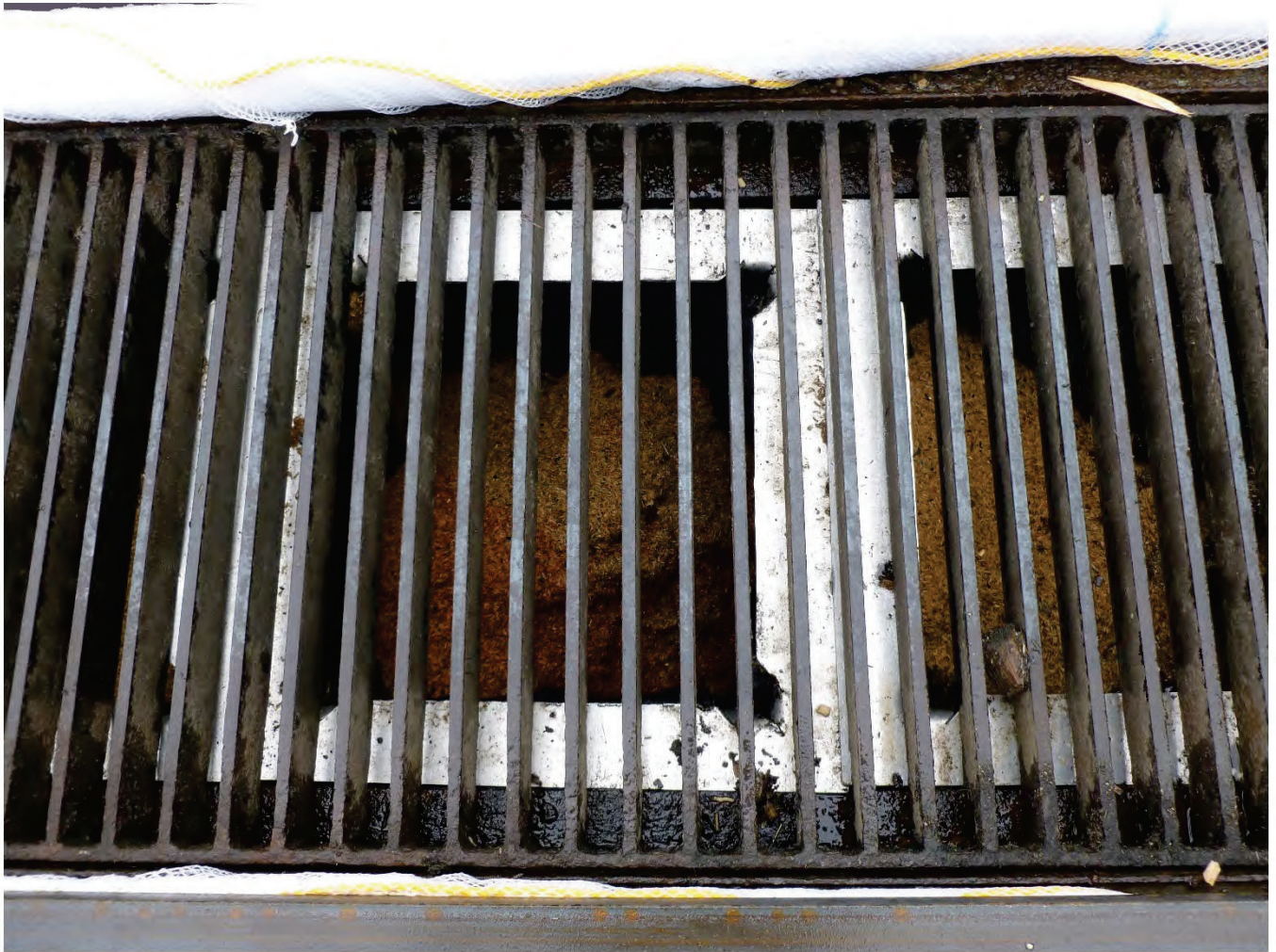
Photo 14 / P1000830 – Catch Basin with Media, close-up
