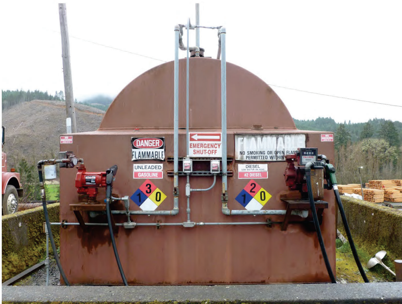
Photo 2 / P1000815 – Gas/Diesel Tank, double-walled, front, facing west
