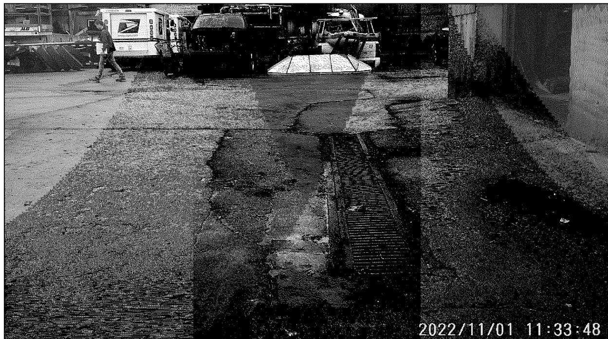
Photograph 13. View, facing east, of the third trench drain at the Facility to the north of the southern garage.
