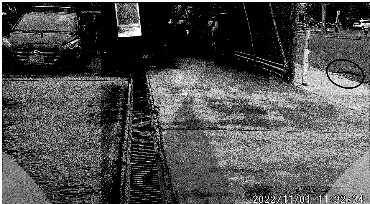
Photograph 12. View, facing east, of the trench drain shown in Photograph 11 and a City of Lowell combined storm sewer drain (red).
