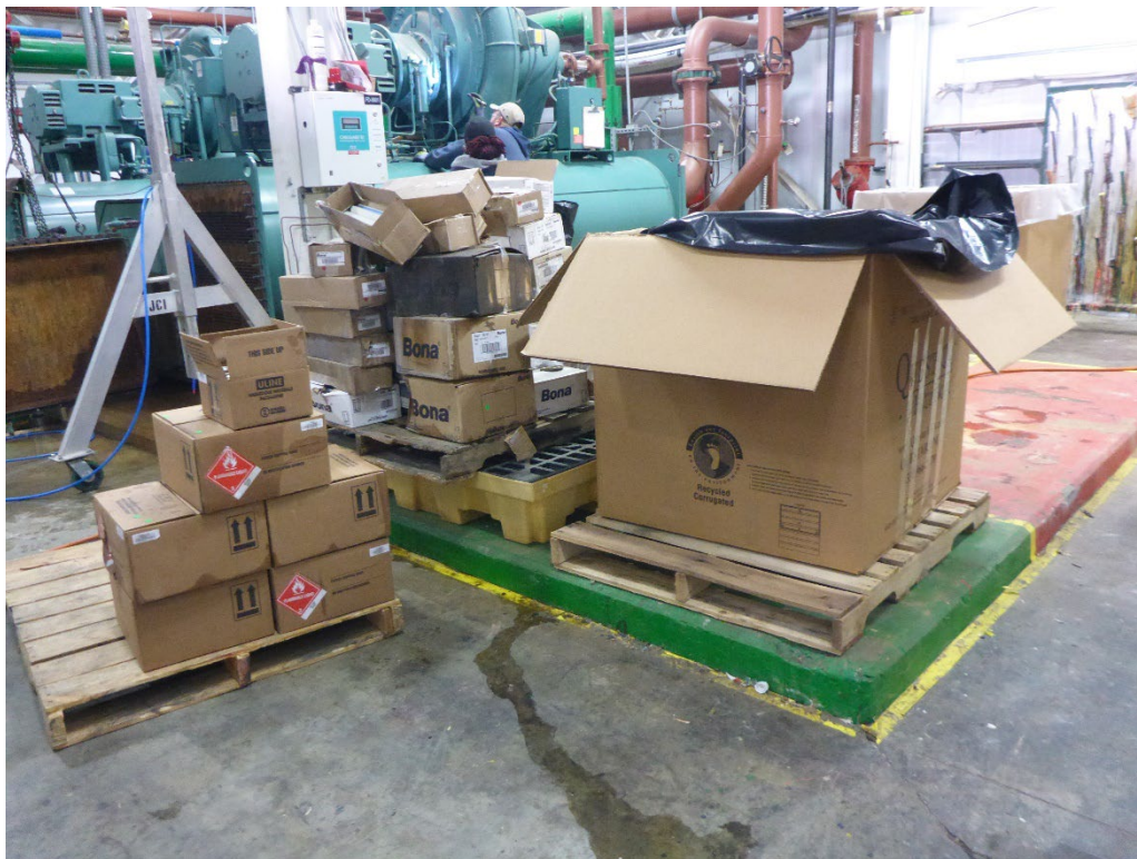
Photo 19: Area within Main CAA where wastes are consolidated according to color-coding system. The cubic yard box and some smaller containers are open. None of the containers are labeled as hazardous waste, marked with an accumulation start date, or identified with an indication of the hazards of their contents.
