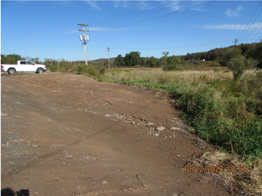
IMG 1617: View facing northeast of area R-2, as defined in the Site's Restoration Plan. This area is directly adjacent to the Unnamed Tributary. The soil in the northwest part of the site, near the toe of the slope, was found to be excessively compact.
