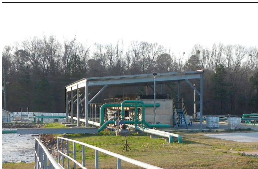
Photo-4. DSM Pretreatment - Covered DAF Unit
