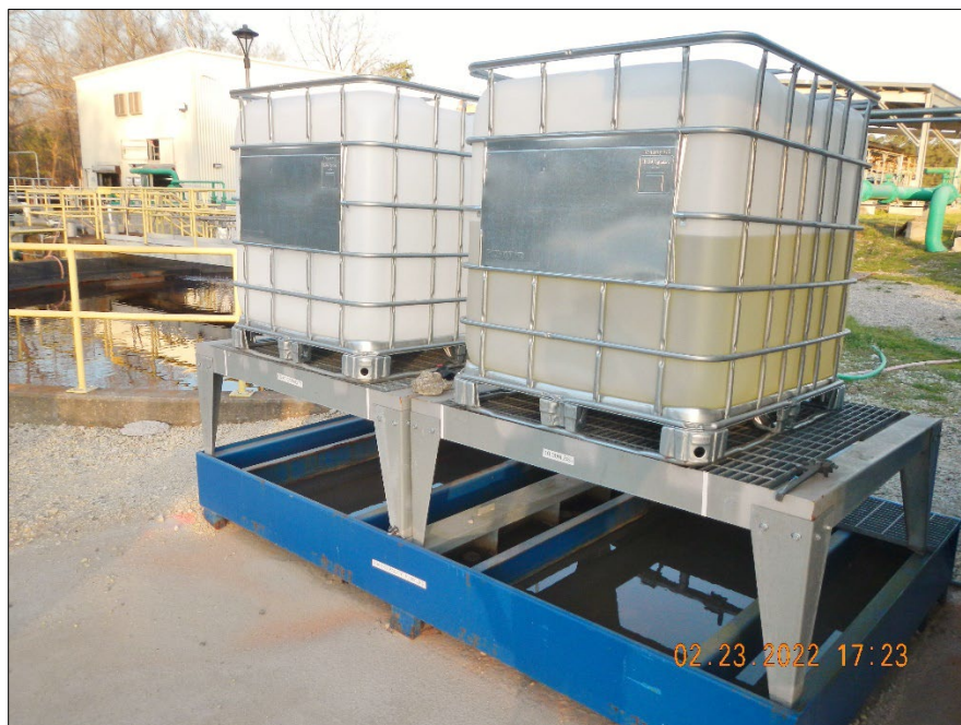
Photo-8. DSM Pretreatment – Coagulant Totes Near Effluent Flume
