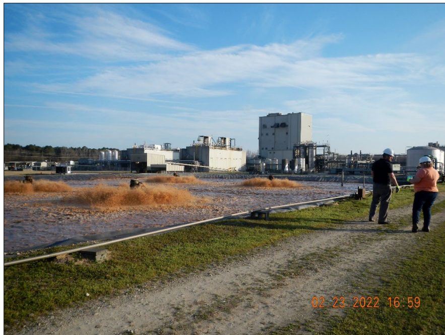
Photo-2. DSM Pretreatment - Influent Equalization Basin with Aerators
