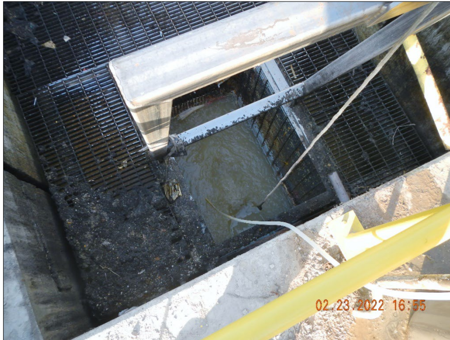
Photo-1. DSM Pretreatment - Influent Pit and Sampling Tube
