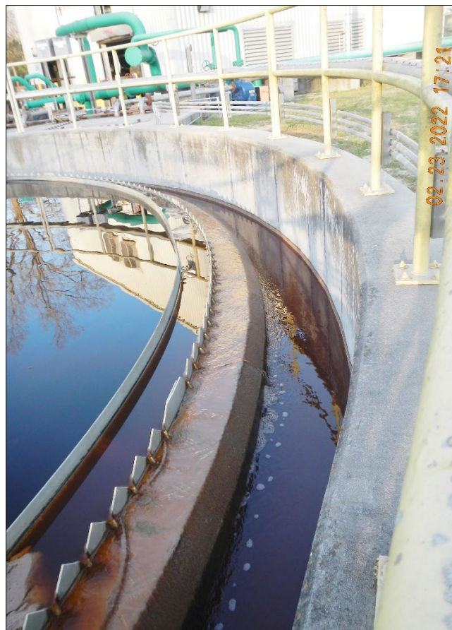
Photo-6. DSM Pretreatment - 12-FT Clarifier Overflow
