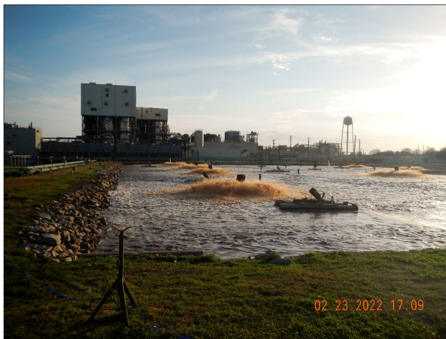
Photo-3. DSM Pretreatment - Aeration Basin
