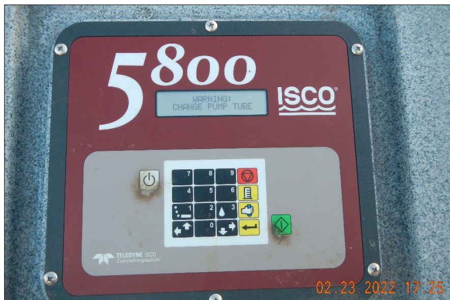
Photo-9. DSM Pretreatment – Effluent Compositor Tube Warning
