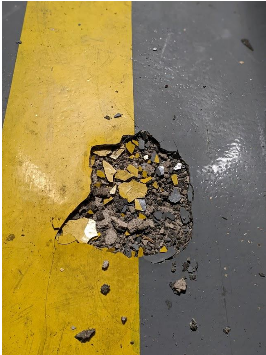
Photograph 1 of 1: Secondary Liner in Hazardous Waste Storage Area
