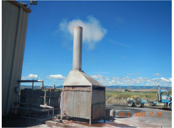
Photo #:14 (DSCN3304) Description: Facing west, photo of the boiler blowdown evaporation tank. Producing steam from evaporating the process water from the deaeration tank.
