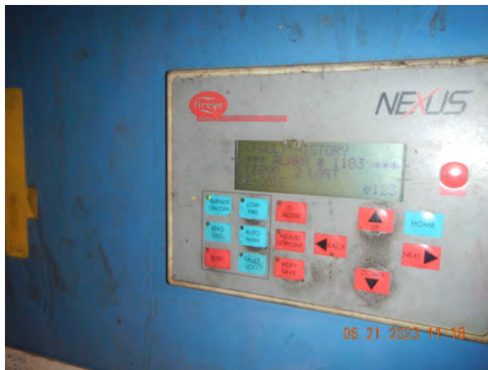
Photo #:20 (DSCN3310) Description: Photo of the Boiler #4 display panel. Showing alarm code for the 02 sensor that has been out and being replaced by Yakima Mechanical.
