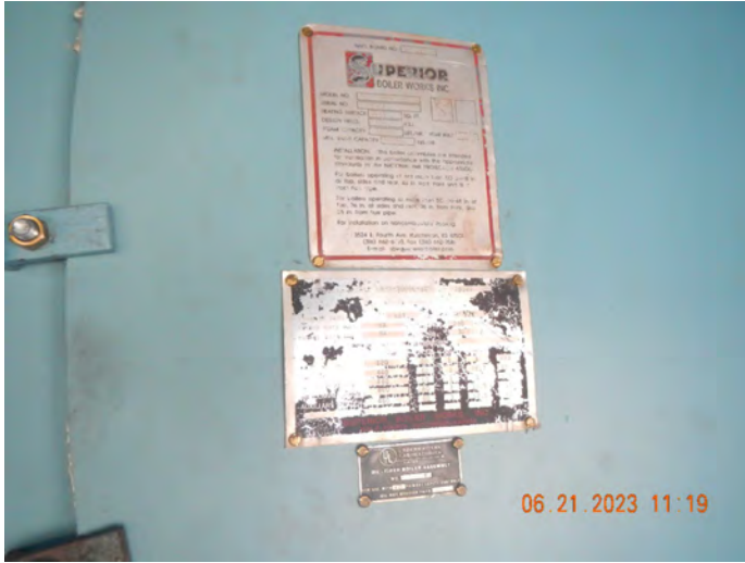
Photo #:21 (DSCN3311) Description: Photo of the Boiler #3 placard.
