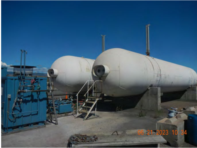
Photo #:13 (DSCN3303) Description: Facing northwest from the “large log yard,” photo of the propane tanks that fuel the Boiler #3 and Boiler #4. Propane is delivered daily (approx), by White Swan Farm Supply.
