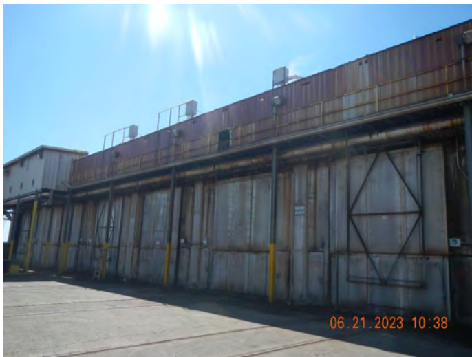
Photo #:15 (DSCN3305) Description: Facing south from the “large log mill,” photo of the kilns (#2-6). Kilns #2, 3, 4, 5 were operating at the time inspection, Kiln #1 was offline to repair the track, Kiln #7 was offline due to maintenance on the steam coil piping.
