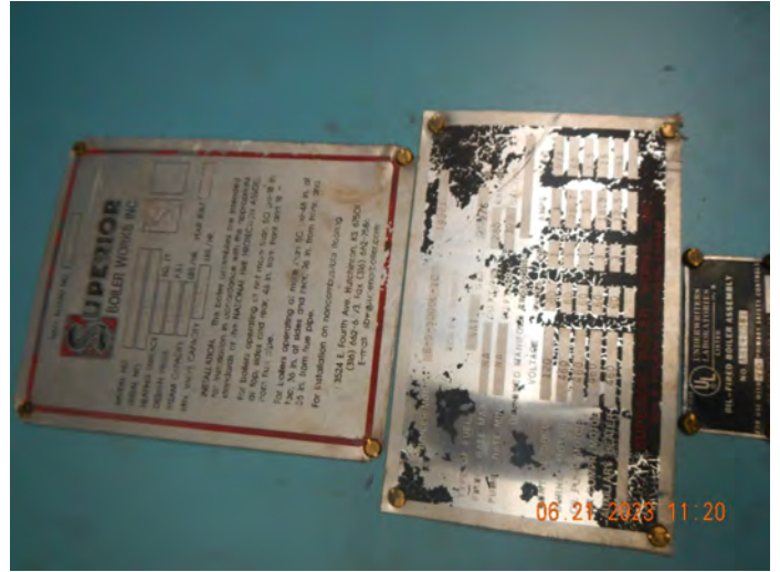
Photo #:22 (DSCN3312) Description: Photo of the Boiler #3 placard.
