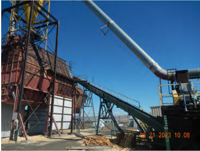
Photo #:05 (DSCN3294) Description: Facing north from the “small log mill,” photo of the dry chip and dry shaving bins and associated conveyors.
