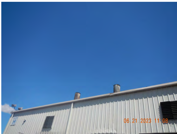
Photo #:19 (DSCN3309) Description: Facing north, photo of the two stacks from Boiler #3 (left) and Boiler #4 (right).
