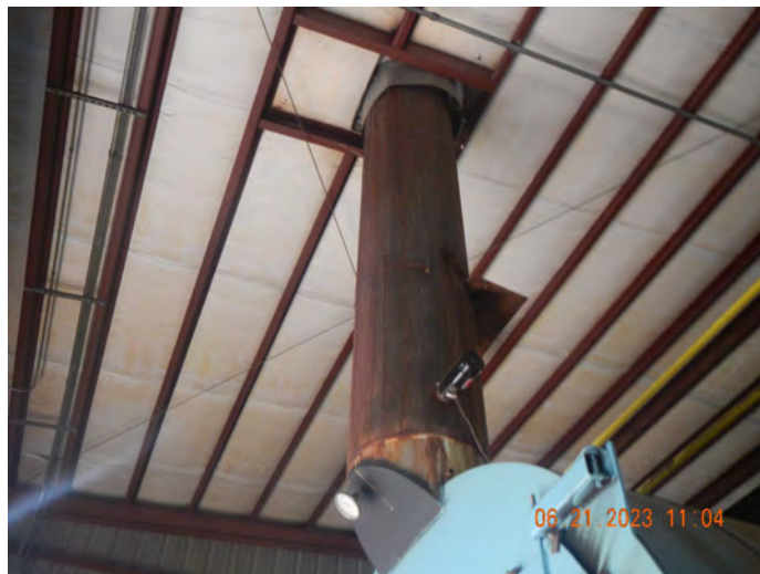
Photo #:18 (DSCN3308) Description: Photo of the Boiler #3 O2 sensor.
