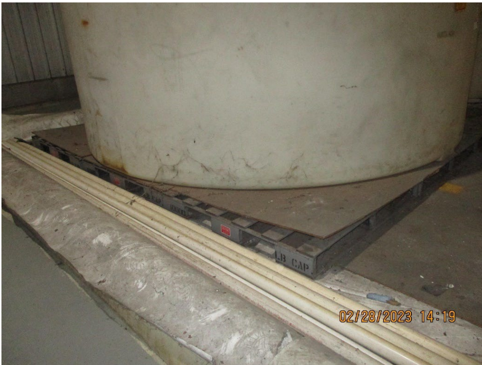
Photograph 10: Metal pallets on which the tanks rest.
