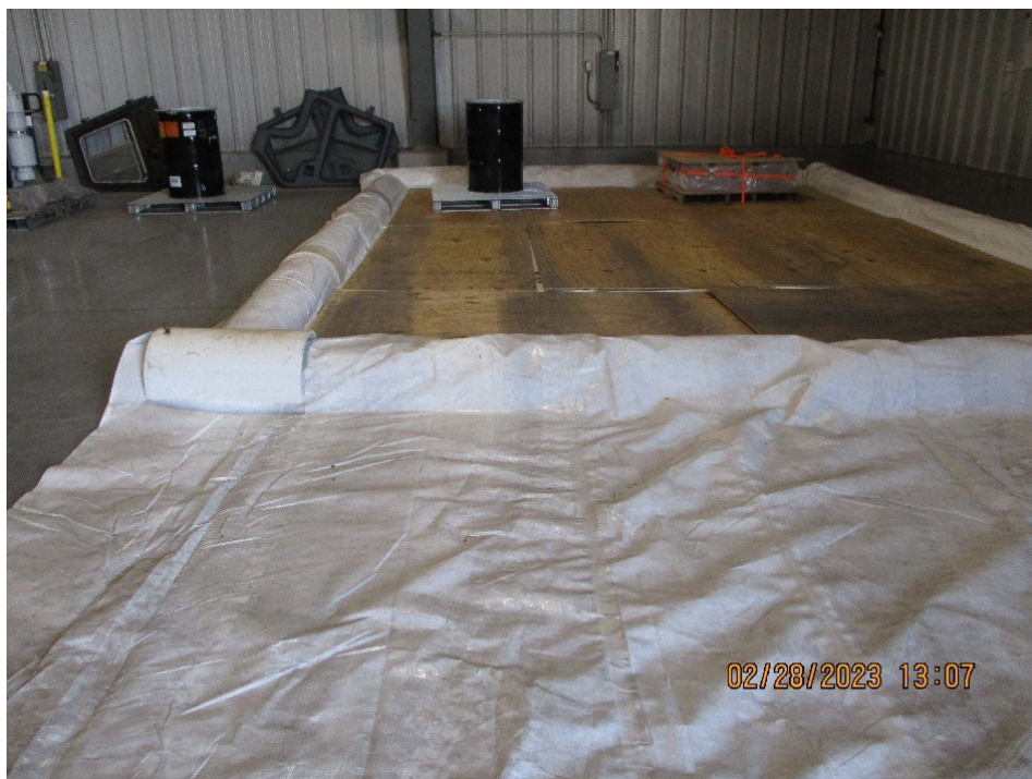
Photograph 3: Example of secondary containment in many areas.
