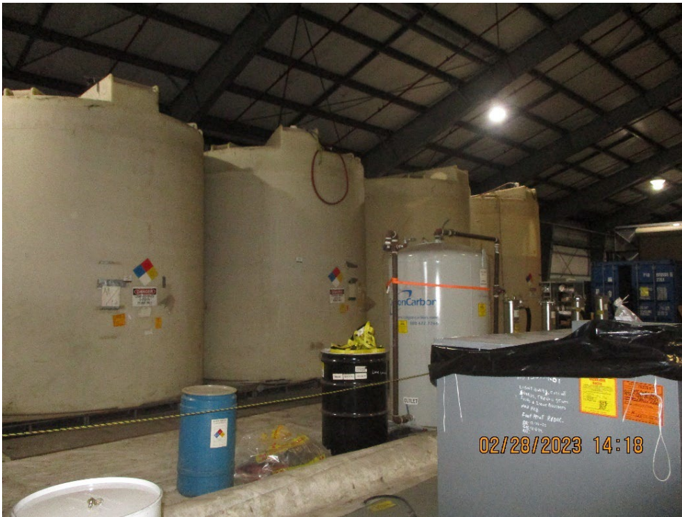
Photograph 9: Four 10,500 hazardous waste storage tank.
