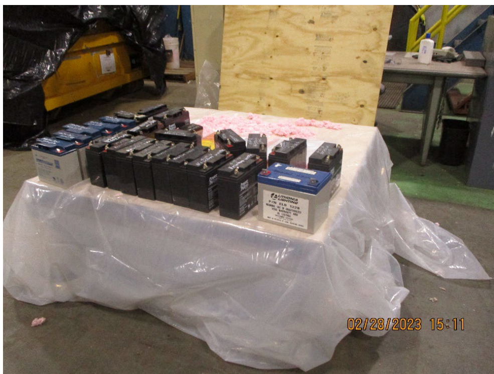
Photograph 16: Battery staging area.
