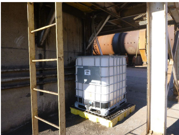
Photograph 14: Used Oil near kilns.
