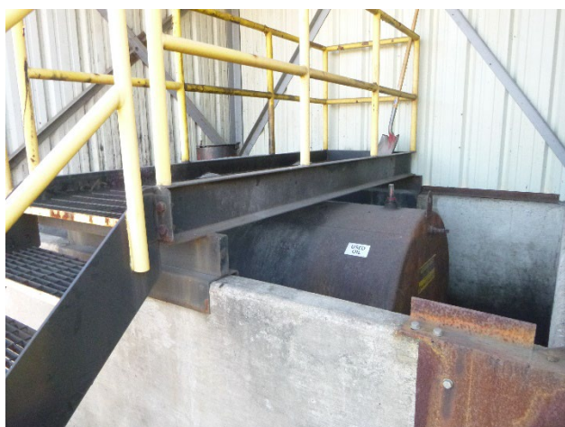
Photograph 20: Used Oil Tank.
