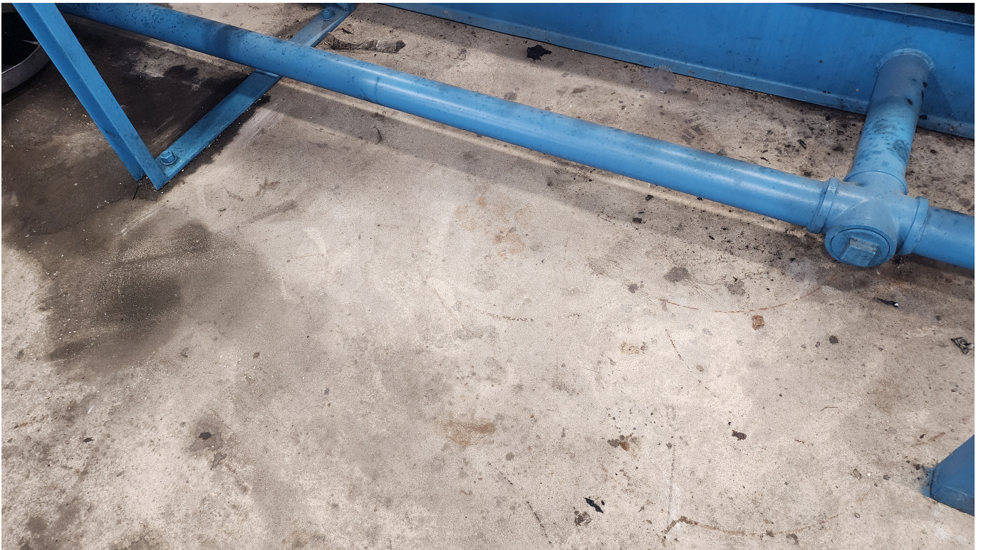
Photograph of oil spills cleaned up provided by Action Oil on 11/18/2024 in response to AOCs
