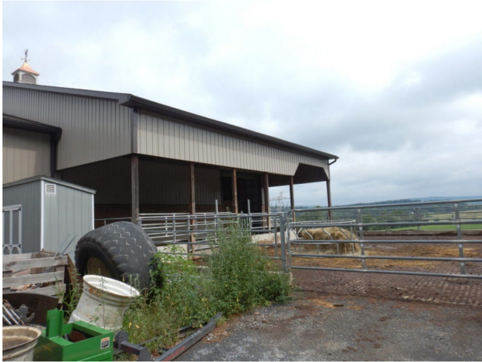
Photograph 21. View of the cattle pen and housing area. Note the manure covering the concrete pad.
