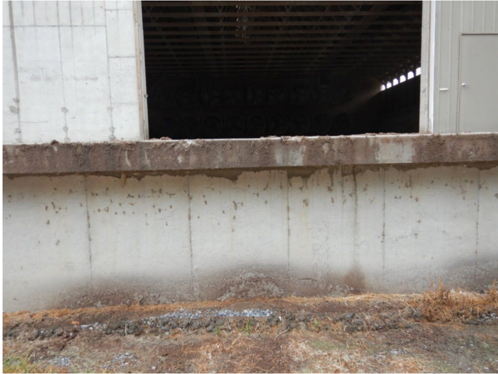
Photograph 9. Close-up view of the edge of the concrete pad on the eastern side of the manure storage building. Note the residual manure accumulated on the edge and the ground below.
