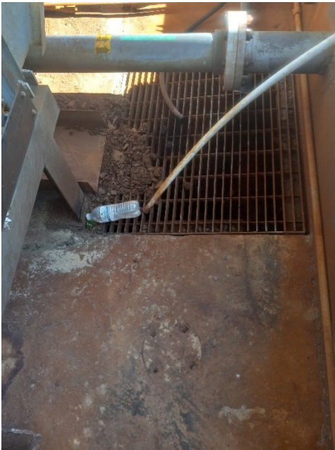
Photograph 63 – IWTP filter cake grate with F019 material
