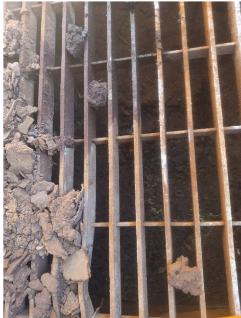
Photograph 64 – IWTP filter cake grate with F019 material and build-up in grate
