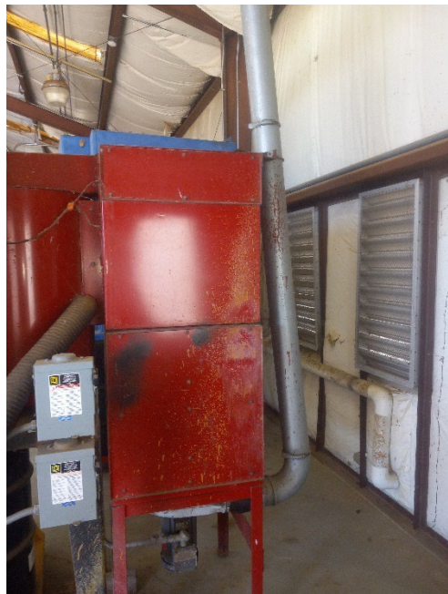
Photograph 60 – 5511 Recycling Center aerosol can crusher ventilation pipe
