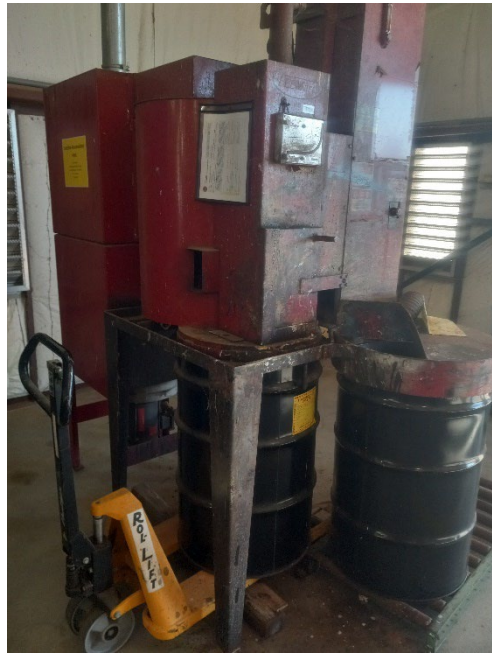
Photograph 58 – 5511 Recycling Center aerosol can crusher
