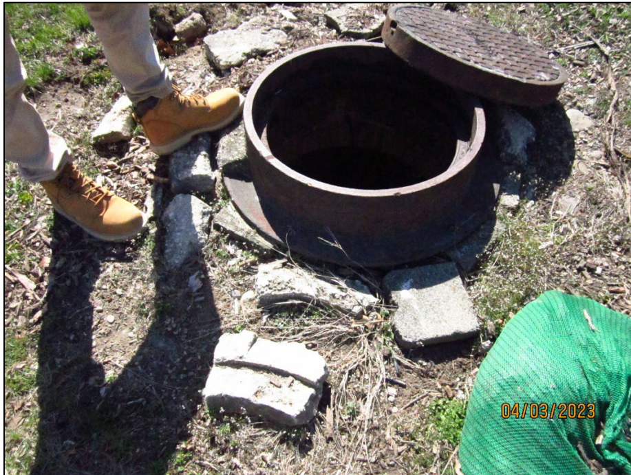
Photograph 18. (IMG_0106) View of the broken manhole located just outside the Plant's southern fence.
