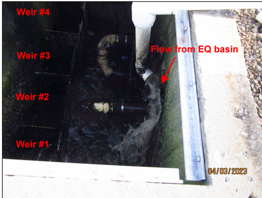
Photograph 8. (IMG_0046) View of flow to the splitter box from the EQ basin. Note the concentration of flow to the first weir leading to Treatment Train #1.
