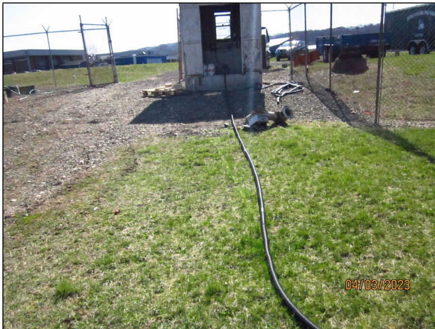
Photograph 14. (IMG_0076) Exterior view, facing South, of sump pump tubing from the digester back to the headworks.
