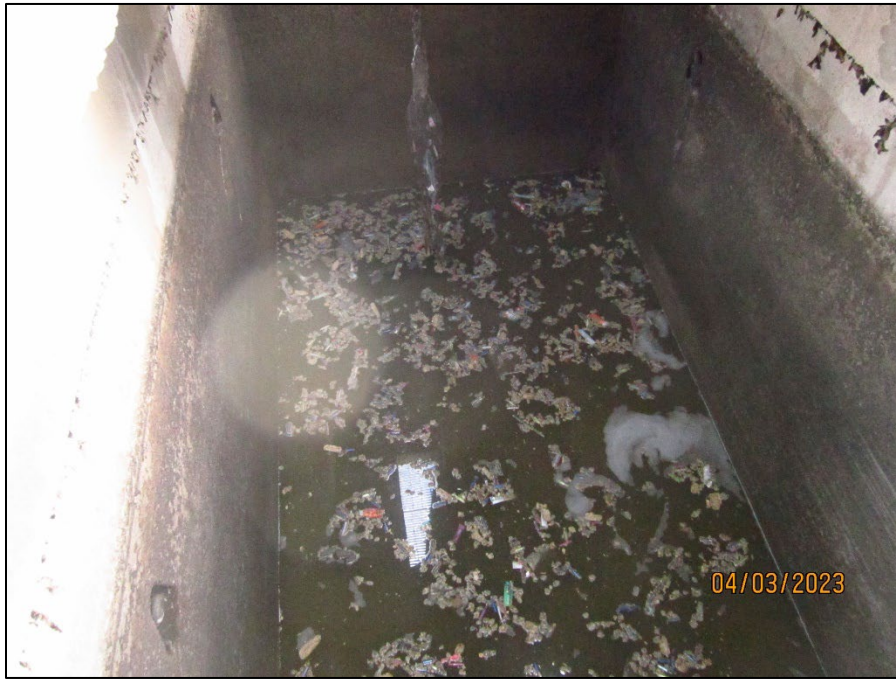
Photograph 7. (IMG_0041) View inside the EQ basin. Note the accumulation of debris.
