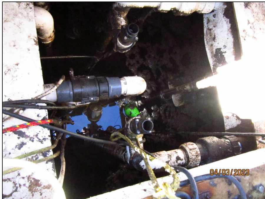
Photograph 10. (IMG_0059) View of aeration chamber in Treatment Train #1. Note the miscellaneous ropes and make-shift rigging.
