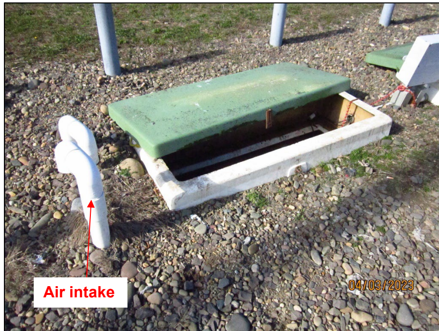
Photograph 9. (IMG_0052) View of the aeration chamber in Treatment Train #1. The external air intake piping did not provide suction at the time of inspection.
