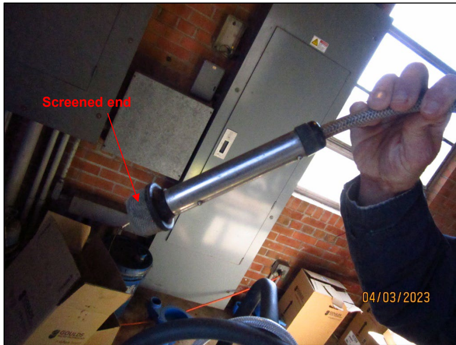
Photograph 15. (IMG_0081) View of effluent sampler strainer with screened end.
