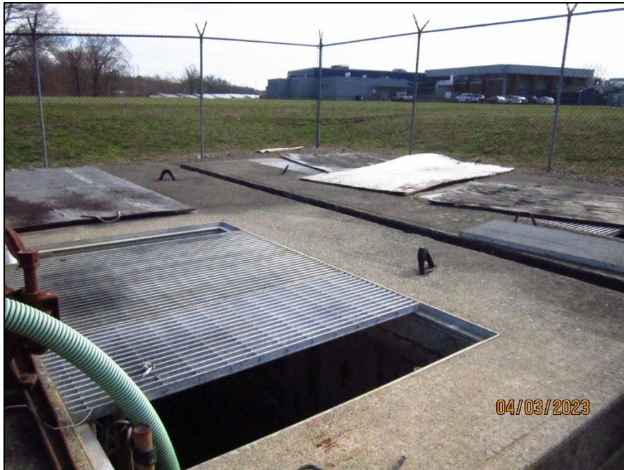
Photograph 6. (IMG_0037) View of the EQ basin. Note the external tubing and plywood coverings.
