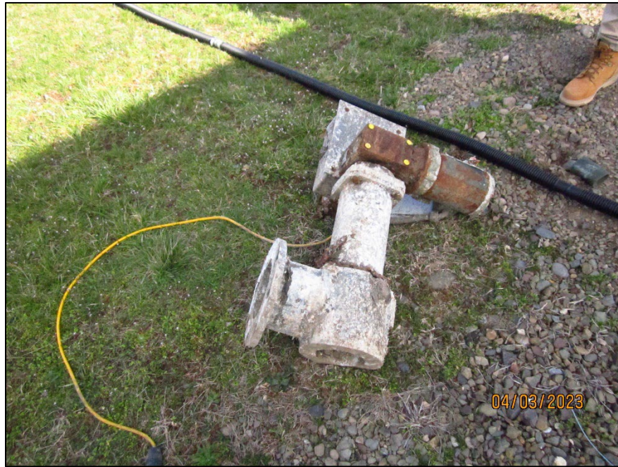
Photograph 3. (IMG_0021) View of the old comminutor laying outside of the influent station. Note there was evidence of submergence.
