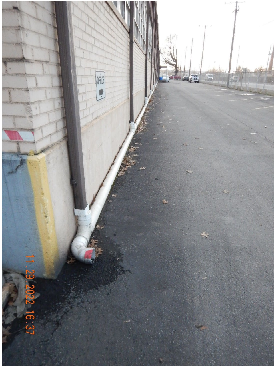
Photo 1. (DSCN5189) Plastic piping connected to multiple roof drains along the northeast side of the West Plant warehouse.
