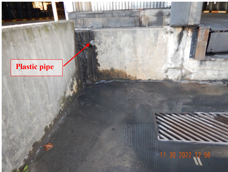
Photo 3. (DSCN5203) Loading dock on the east side of the West Plant warehouse, with stormwater flowing from a plastic pipe on 11/30/2022. Carbon accumulation was observed.
