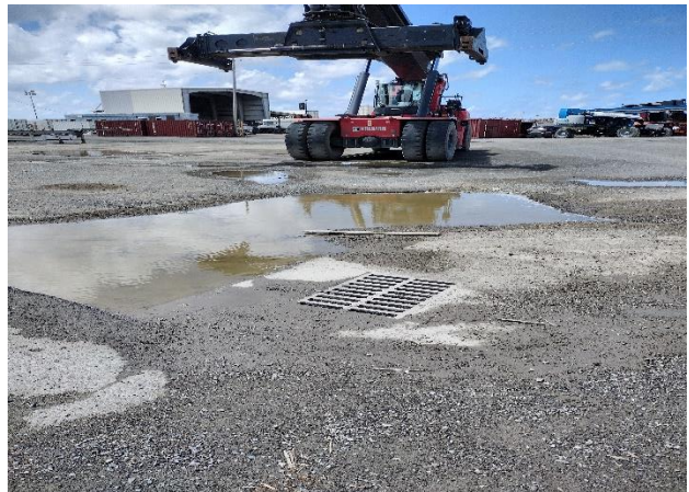
IMG 2816 -Retention area where stormwater runoff from the unpaved south section of CommUserArea 1 is collected and drained-off. Inlets are unprotected.
