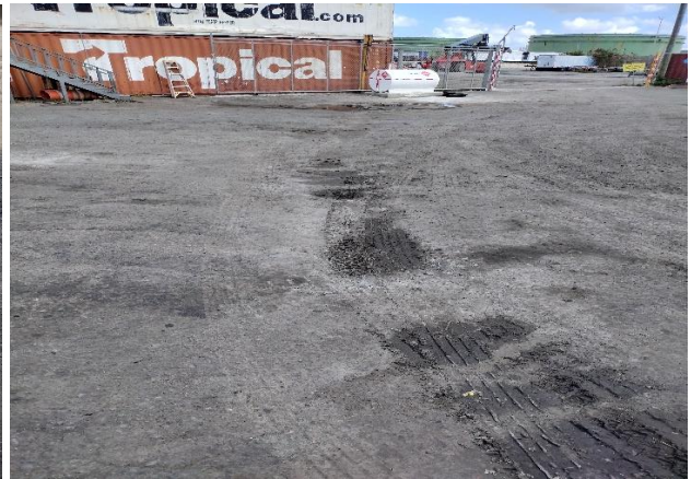
IMG 2768 -Close-up of stormwater runoff path that appeared saturated with oil patches along the stormwater path towards the stormwater catch basin.
