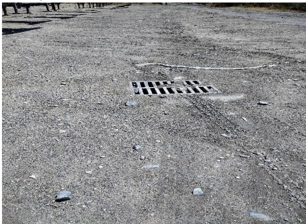
IMG 5058 -Partially clogged storm inlet midway of unpaved south section of CommUserArea 1.
