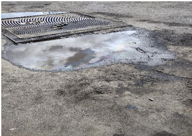
IMG 8118 -View of the large stormwater catch at low point in the yard of the maintenance shed. Oil spills patches next to the puddles observed.
