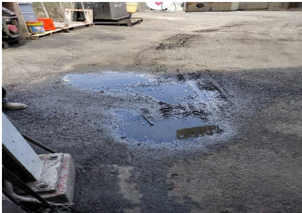
IMG 1616 -Stormwater runoff path observed from front of the shed flowing downhill towards a large stormwater catch basin at the low-point in the yard.
