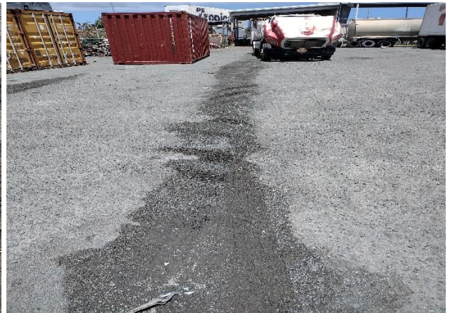
IMG 0111 -Evidence of stormwater runoff flow path from rear side of the maintenance shed, that runs across paved yard area.
