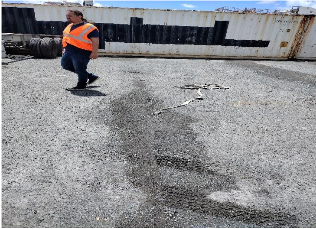
IMG 6966 -Flow path of stormwater flow in the rear yard area of the maintenance shed.
