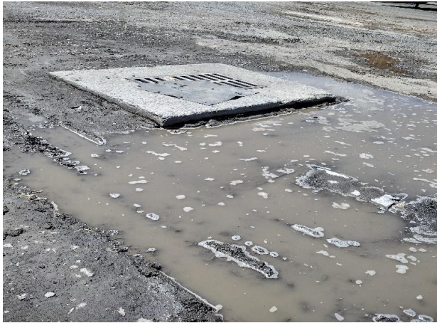
IMG 6258 -Storm inlet and road surface about inlet is deteriorated, and unmaintained. Debris clogging metal grate.
