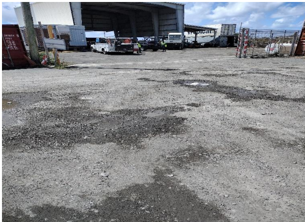
IMG 0179 -Sloped entrance into maintenance shed, where Tropical's vehicle fleet and equipment are regularly serviced. Potential for transport of sediments and gravel into stormwater catch basin.
