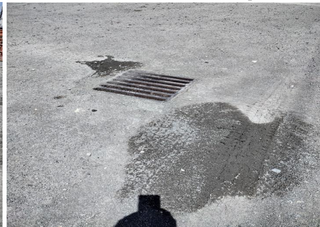
IMG 3660 -Accumulated sediment at base of sloped entrance into the Facility's maintenance shed area. Storm inlet unprotected from transport of sediment by stormwater runoff into stormwater catch basin.
