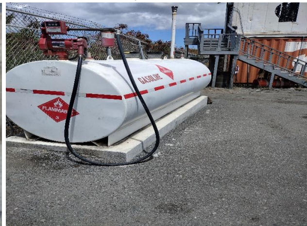
IMG 9911 -Closeup of fueling terminal unit with no containment around the system. Oil-soaked spot next to the tank, and exposed to stormwater runoff.
