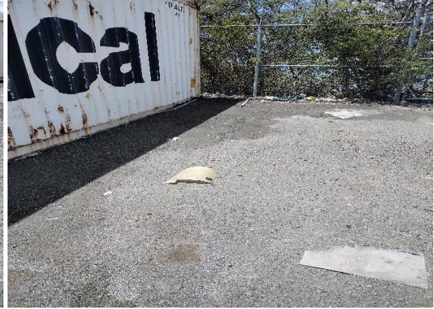
IMG 1793 -Evidence observed that stormwater flow within the rear yard area drains off at the western fence line of the Facility.
