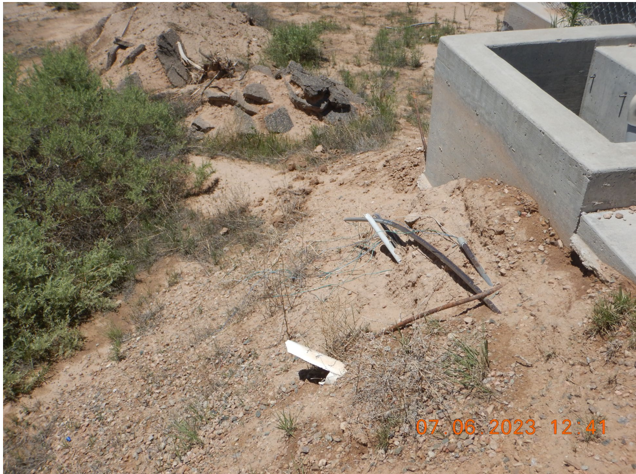
View of a portion of the electrical wiring that has been severed. (DSCN 2563). Photographed by D. Esparza.
