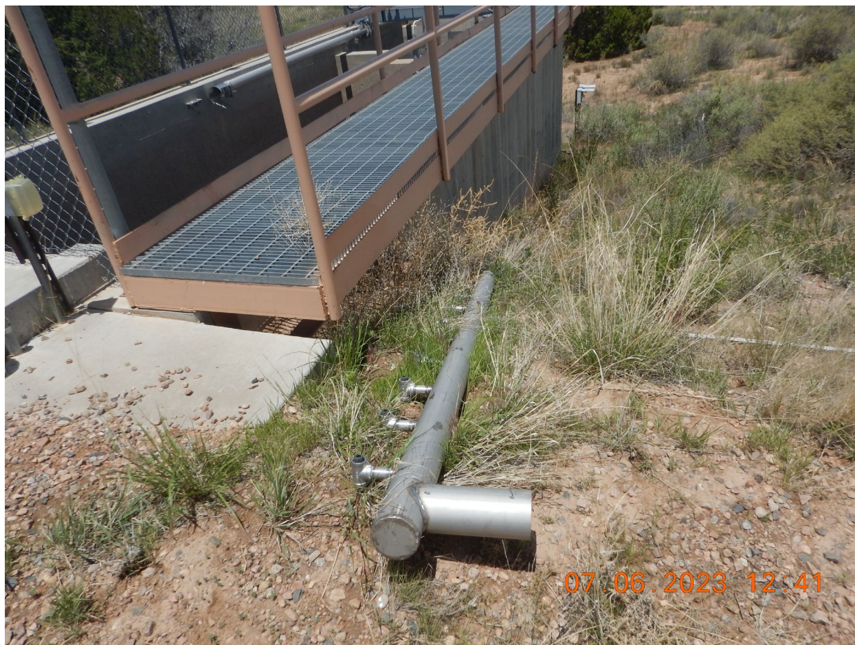
View of some of the associated treatment equipment that has been removed. (DSCN 2562). Photographed by D. Esparza.
