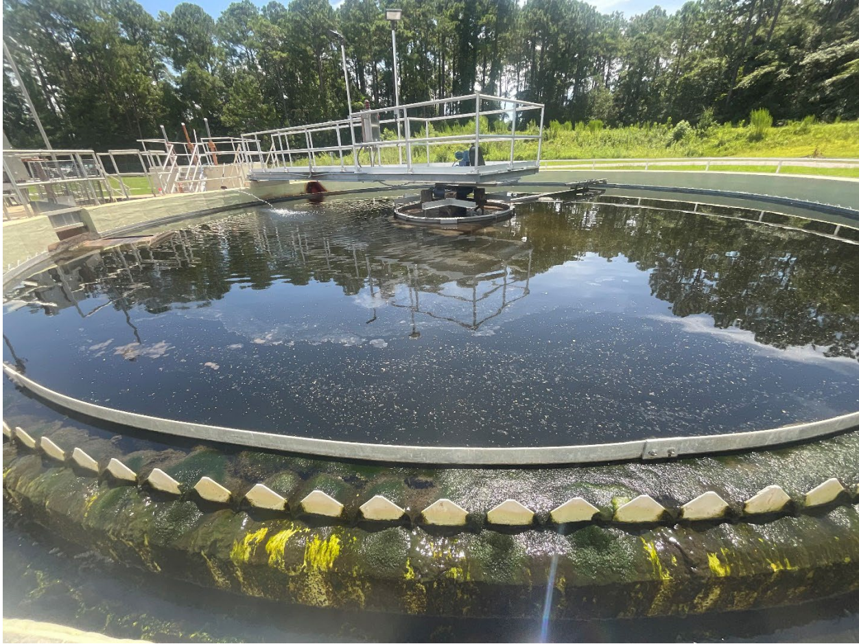
Figure 3 – Presence of Grit in Clarifier and Algae Growth on Weir Plates
