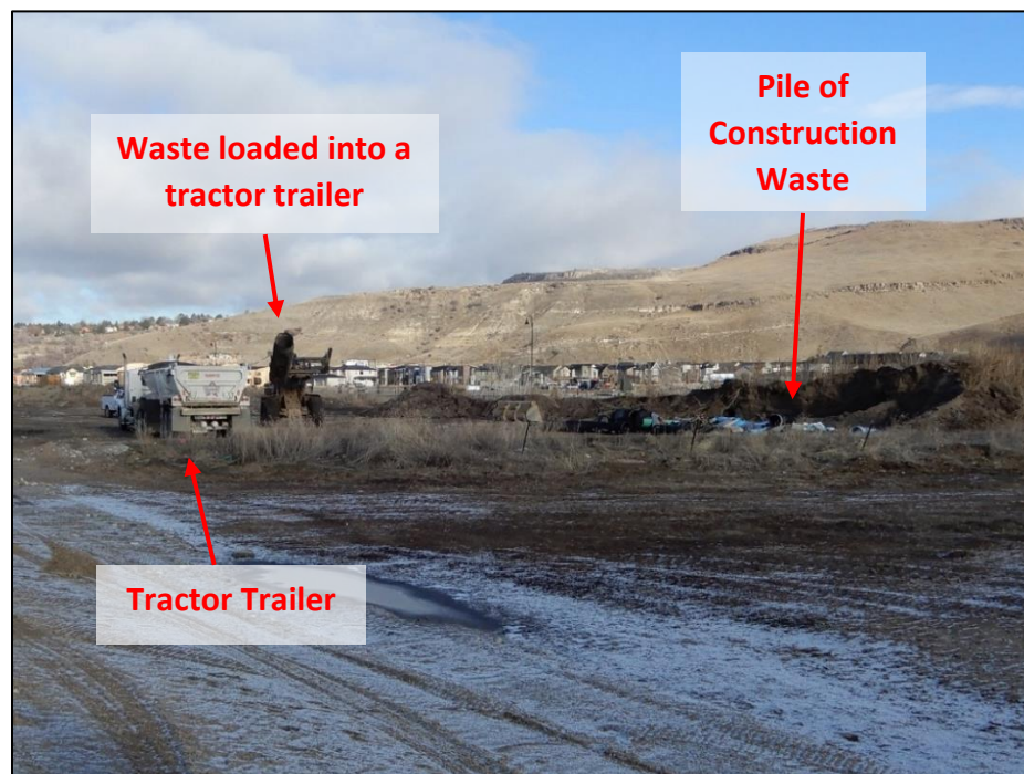
Photograph 6. View, facing northwest, of a pile of uncontained construction waste and debris. At the time of the inspection, the waste was actively being loaded into a tractor trailer.
