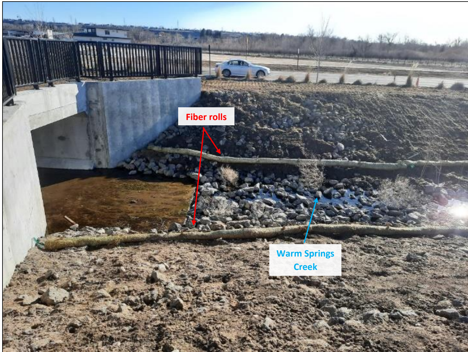
Exhibit 4. View, facing south, of Warm Springs Creek west of East Millbrook Way. The fiber rolls were moved downgradient of the hydro seeded area along the creek. The image was sent to the Inspection Team from Kyle Terrell, on 3/2/2021.
