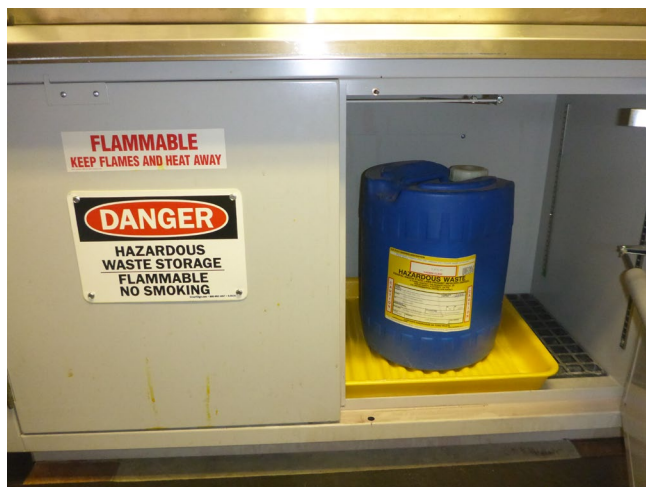
Photo 2: One 5-gallon container of D001, D022, F003, F005, P020 hazardous waste in the Laboratory CAA.
