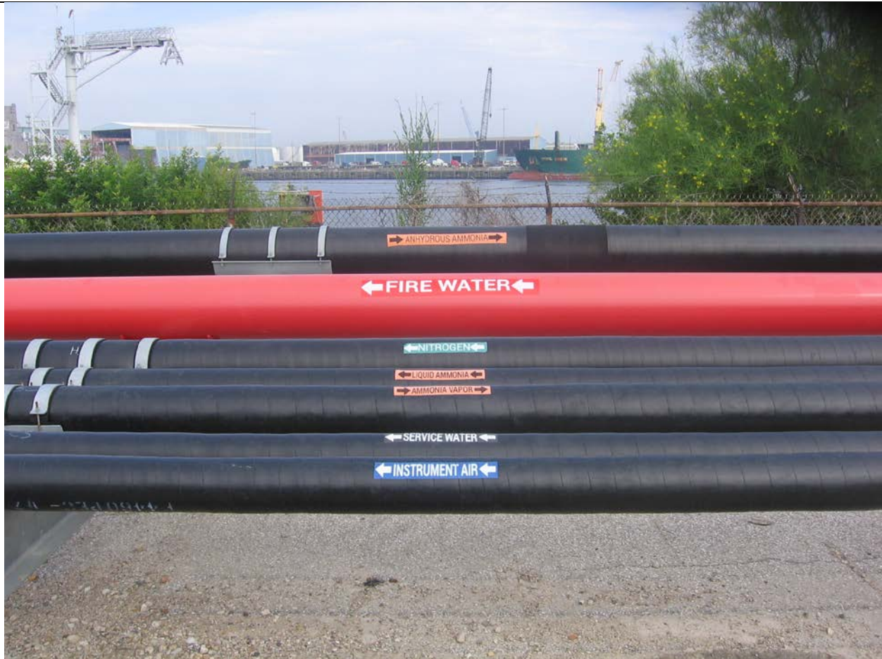
Piping Near Ammonia Tanks Nos. 100 & 101 (Worse Case Scenario)
