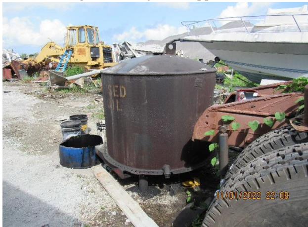
IMG 769- Container in which the Facility's used oil is collected and stored on-site. Improper housekeeping conditions observed and documented.
