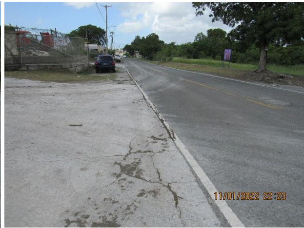
IMG 782- Evidence of track-out of pollutants from Facility and into the public road. Path of stormwater runoff leaving the Facility from upper entrance/exit.
