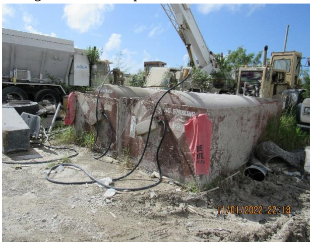
IMG 772- Facility's fueling terminal situated in path of stormwater flow. No containment in area where vehicles are staged for fueling service.
