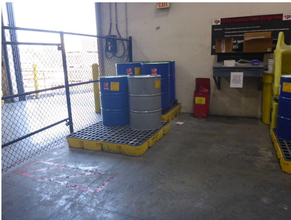
Photo 7: Six 55-gallon drums on portable secondary containment pallets in the near corner immediately to the left inside the entrance to the caged CAA.
