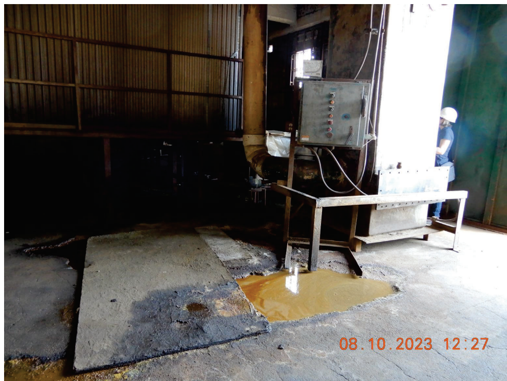
Photo 3. Liquid on warehouse floor near acid rinse area. Acid tank is visible in the background. (DSCN0725.JPG)
