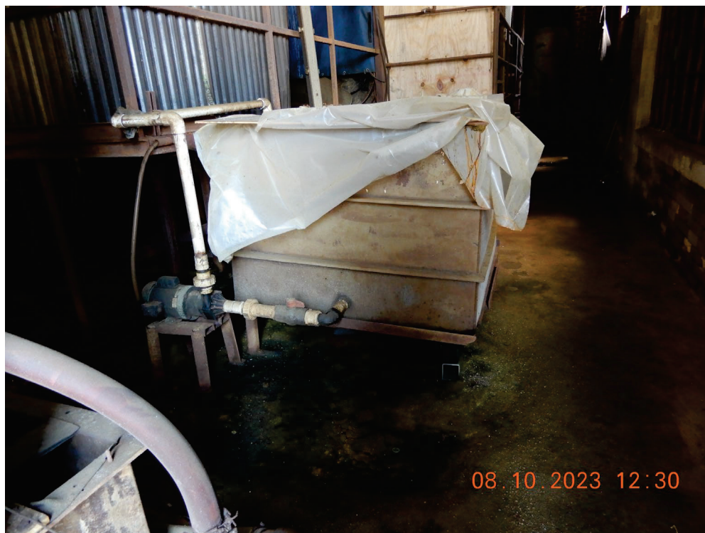
Photo 4. Poly tank containing acid rinse solution. Tank was covered with a plywood sheet as a cover. (DSCN0726.JPG)
