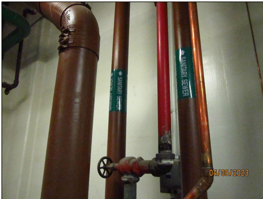
Photograph 2. IMG_0008.JPG View of a large sanitary sewer line at the North Energy Plant. Note the two smaller sanitary sewer sump discharge lines were reported to lead to the City of Baltimore sanitary sewer system.
