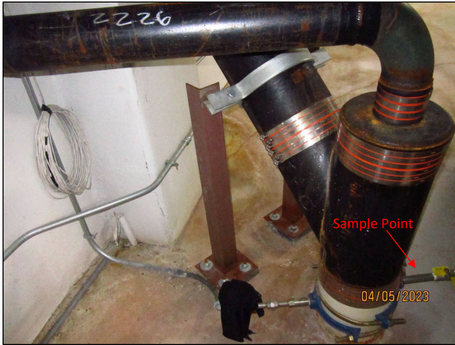
Photograph 7. IMG_016.JPG View of the cooling tower sampling location for Outfall 002 (lower right corner).
