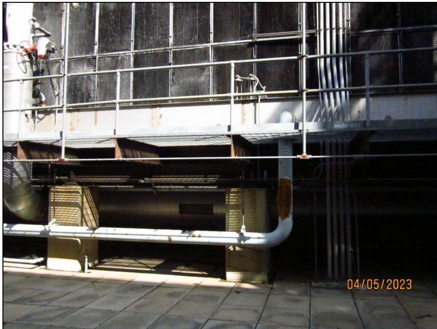
Photograph 10. IMG_022.JPG View of the cooling tower reservoir in the South Energy Plant.
