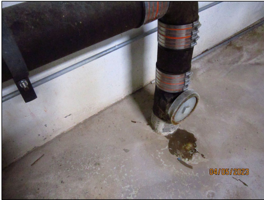
Photograph 9. IMG_019.JPG View of the sump discharge line in the South Energy Plant. The pipe was described as going through the basement floor and connecting to the sanitary sewer system.
