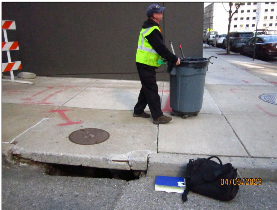
Photograph 4. IMG_0013.JPG Exterior view of the city curb inlet on the southwestern corner of Wolfe Street. Note Outfall 001 is located underneath the manhole on the sidewalk; however, it appeared that samples were collected through the curb access.
