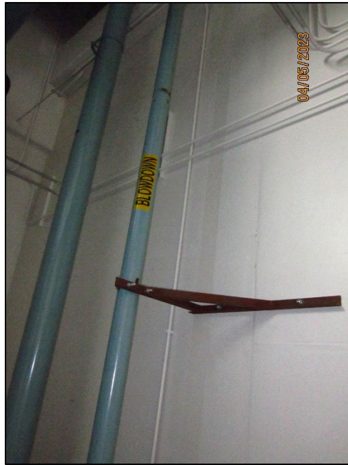
Photograph 5. IMG_020.JPG View of light blue cooling tower blowdown pipes in the South Energy Plant.
