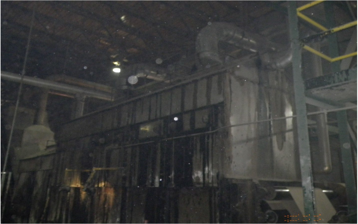
5. Enclosed Paper Saturator Line 1 – Warrior Roofing – 7/19/22
