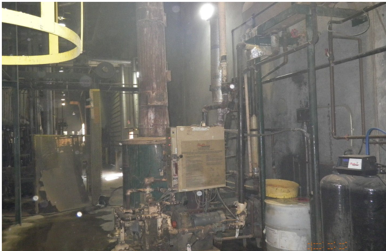
4. Process Steam Generator – Warrior Roofing – 7/19/22
