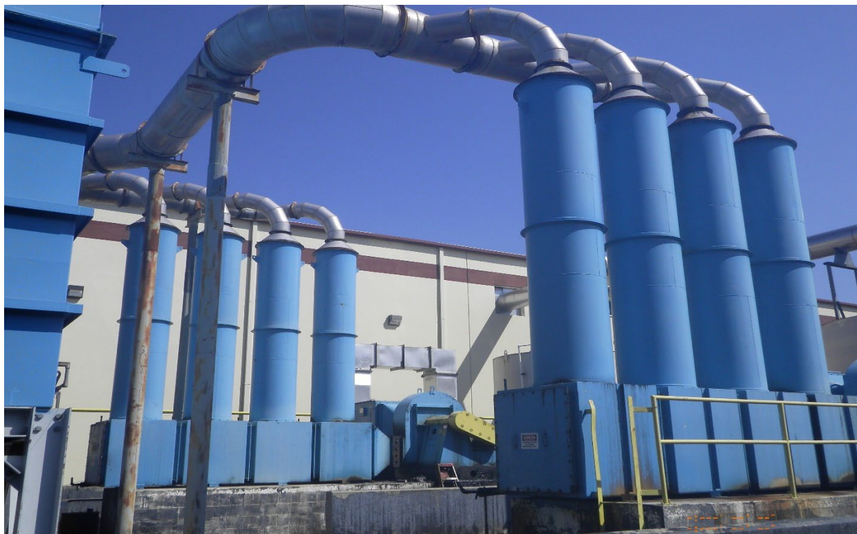
15. Two CECO Air Filters – Warrior Roofing – 7/19/22
