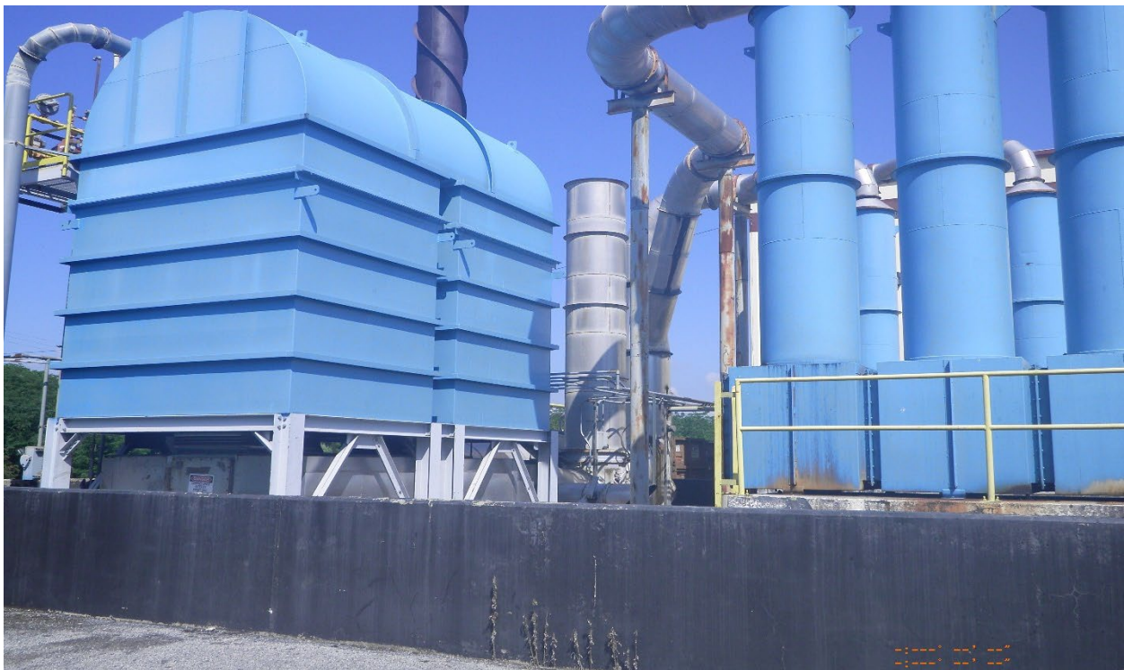
20. Regenerative Thermal Oxidizer Bypass Stack – Warrior Roofing – 7/19/22
