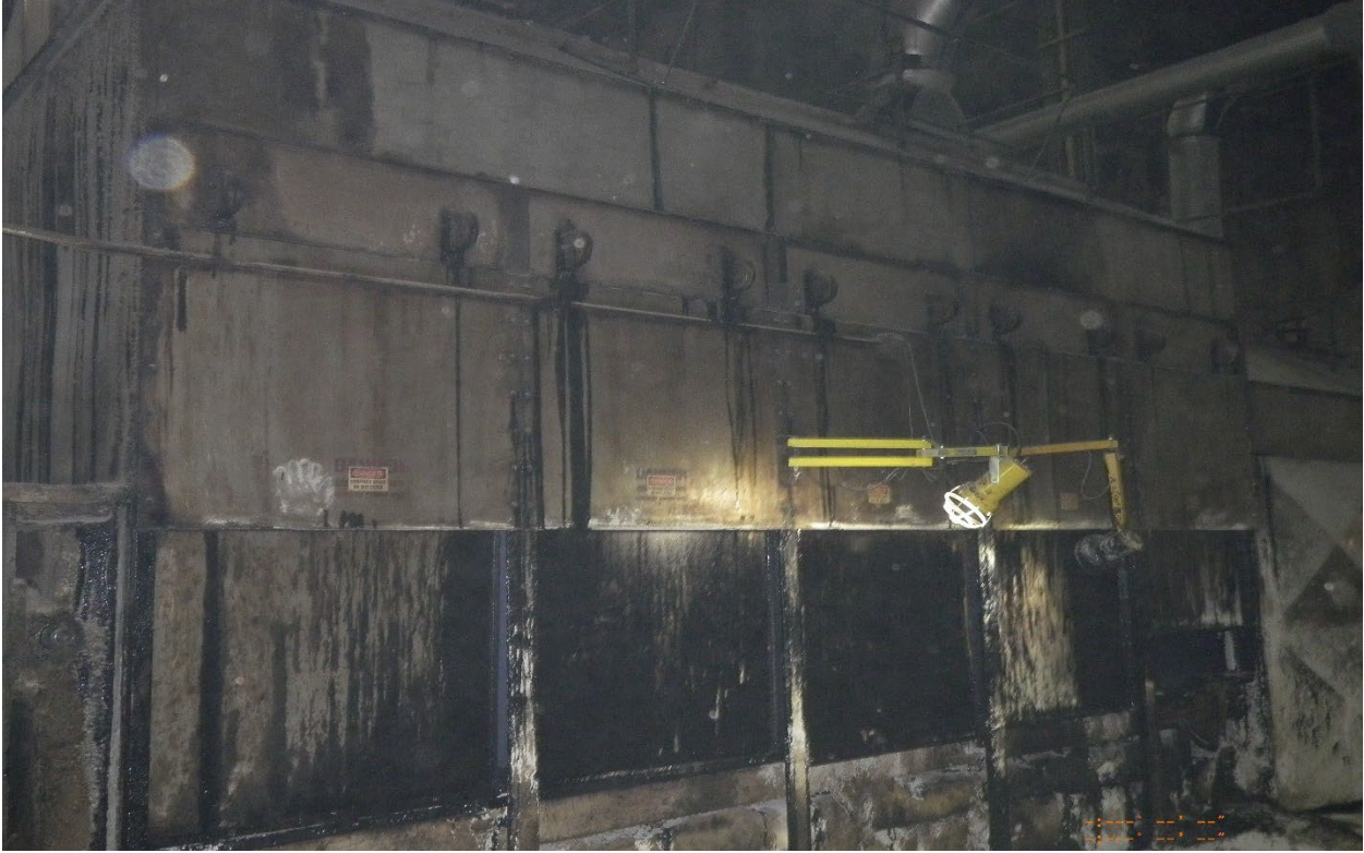
7. Enclosed Paper Saturator Line 2 – Warrior Roofing – 7/19/22
