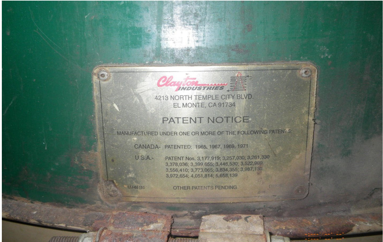
3. Steam Generator Nameplate – Warrior Roofing – 7/19/22
