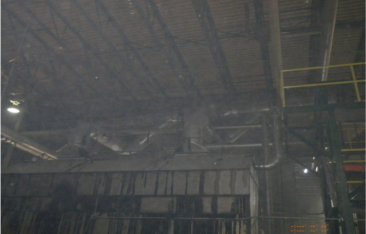
8. Vapor Collection Ductwork above Saturator – Warrior Roofing – 7/19/22
