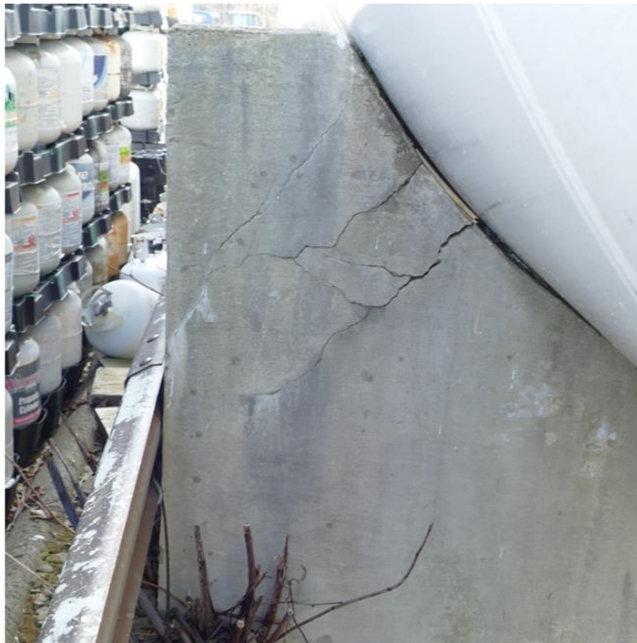
Tank support system in poor repair.
