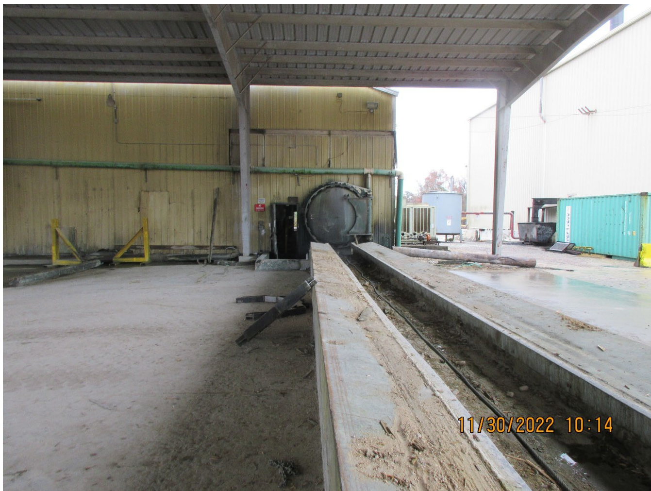
Photo 1 – Rail system and concrete secondary containment system outside of west end of treatment tank
