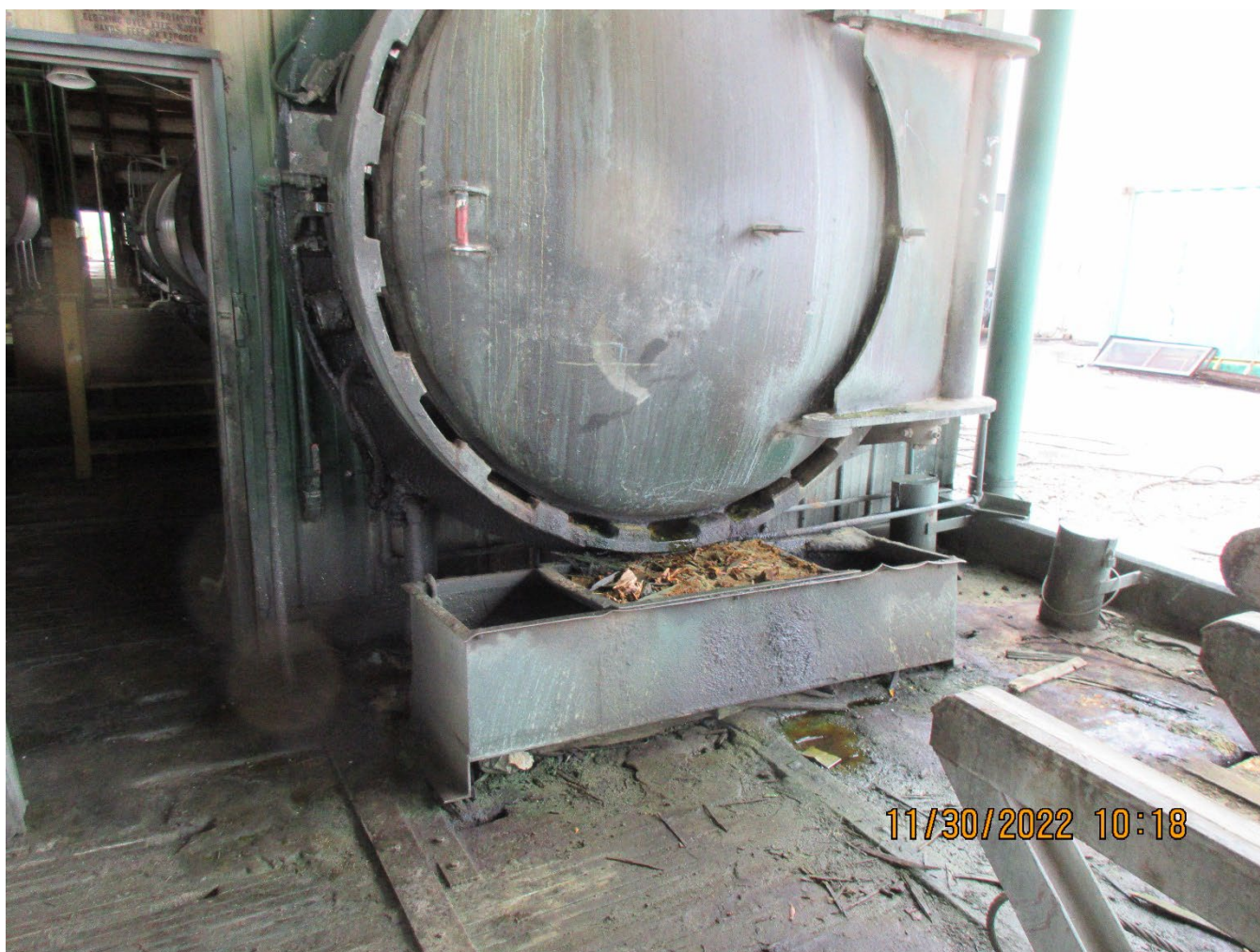
Photo 2 – West end of treatment cylinder and debris catch basin
