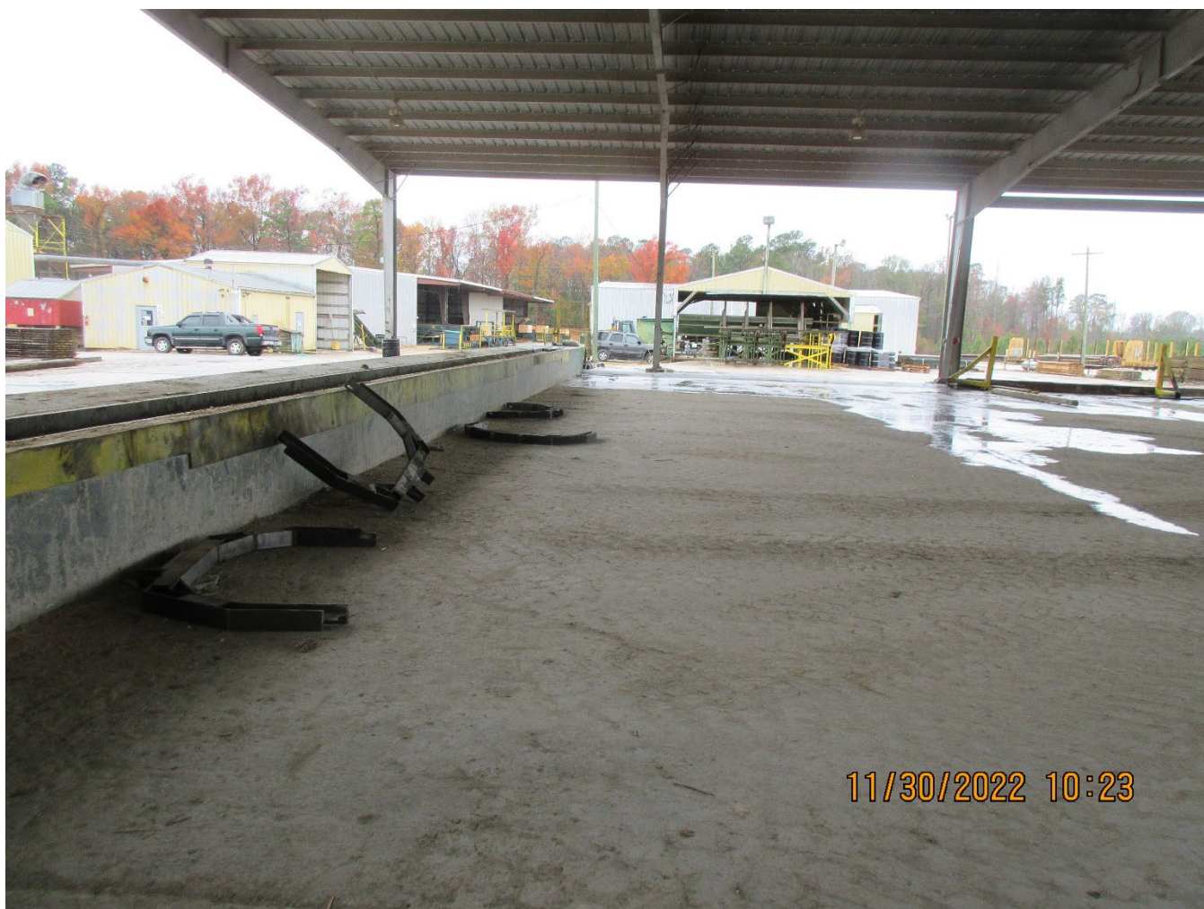
Photo 3 – Rail system and concrete catch basin/drip pad on west end of drip pad. Staging area on right side of drip pad in photo.
