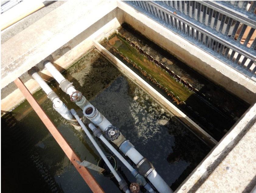
7: DSCN0766 Description: Clarifier weir Location: Wastewater treatment plant Camera Direction: down Date/Time: 4/1/2025 14:44
