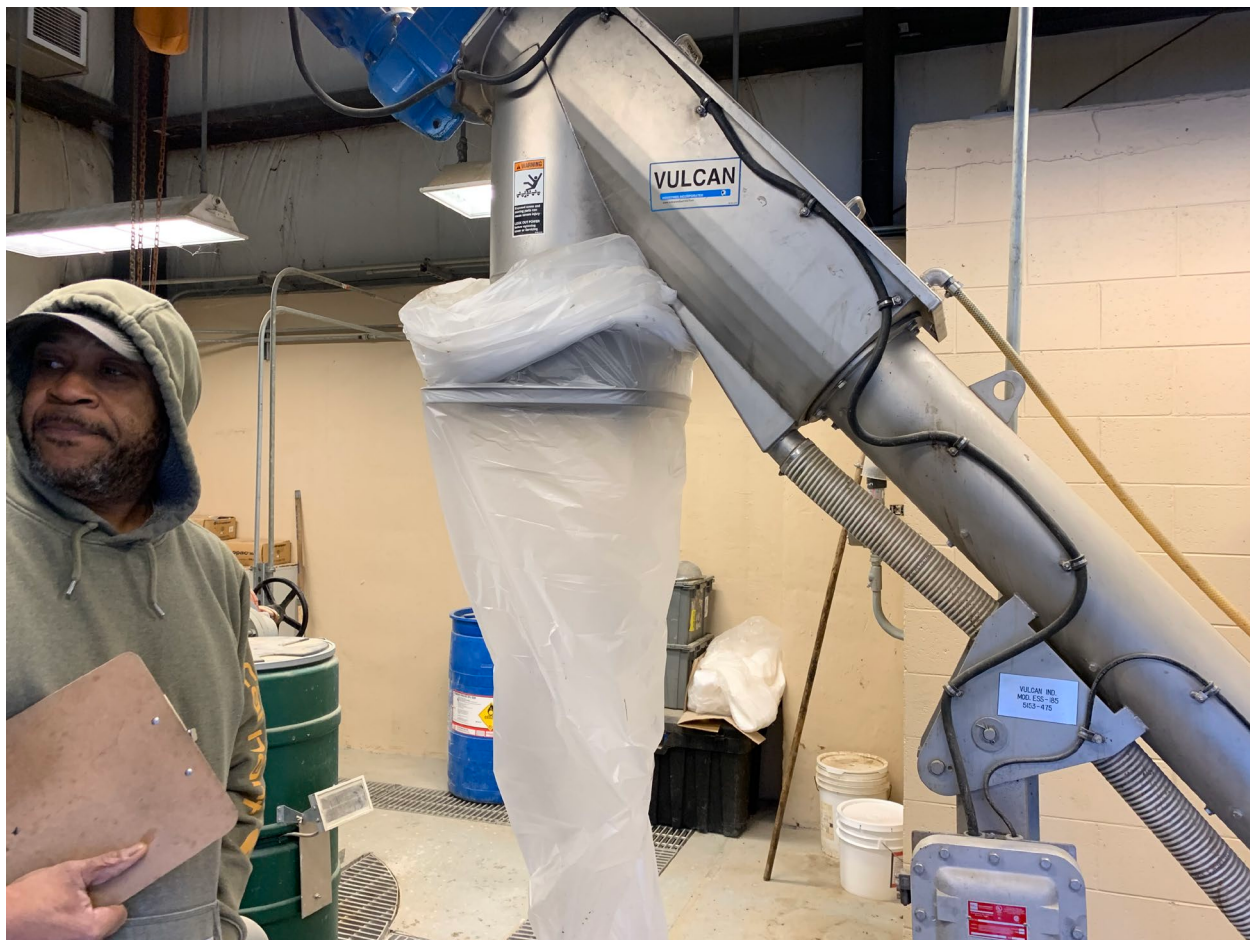
View of the grit bagging system within the headworks. (IMG_0217) (09:15 AM :01/18/2024). Photographed by D. Esparza
