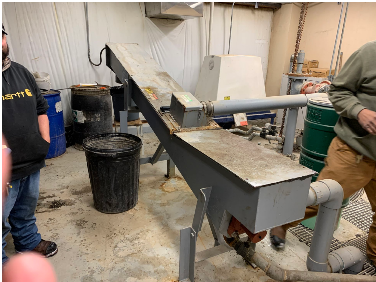
View of one (1) of the WWTP two (2) pieces of process equipment associated with the headworks. (IMG_0216) (09:14 AM:01/18/2024). Photographed by D. Esparza
