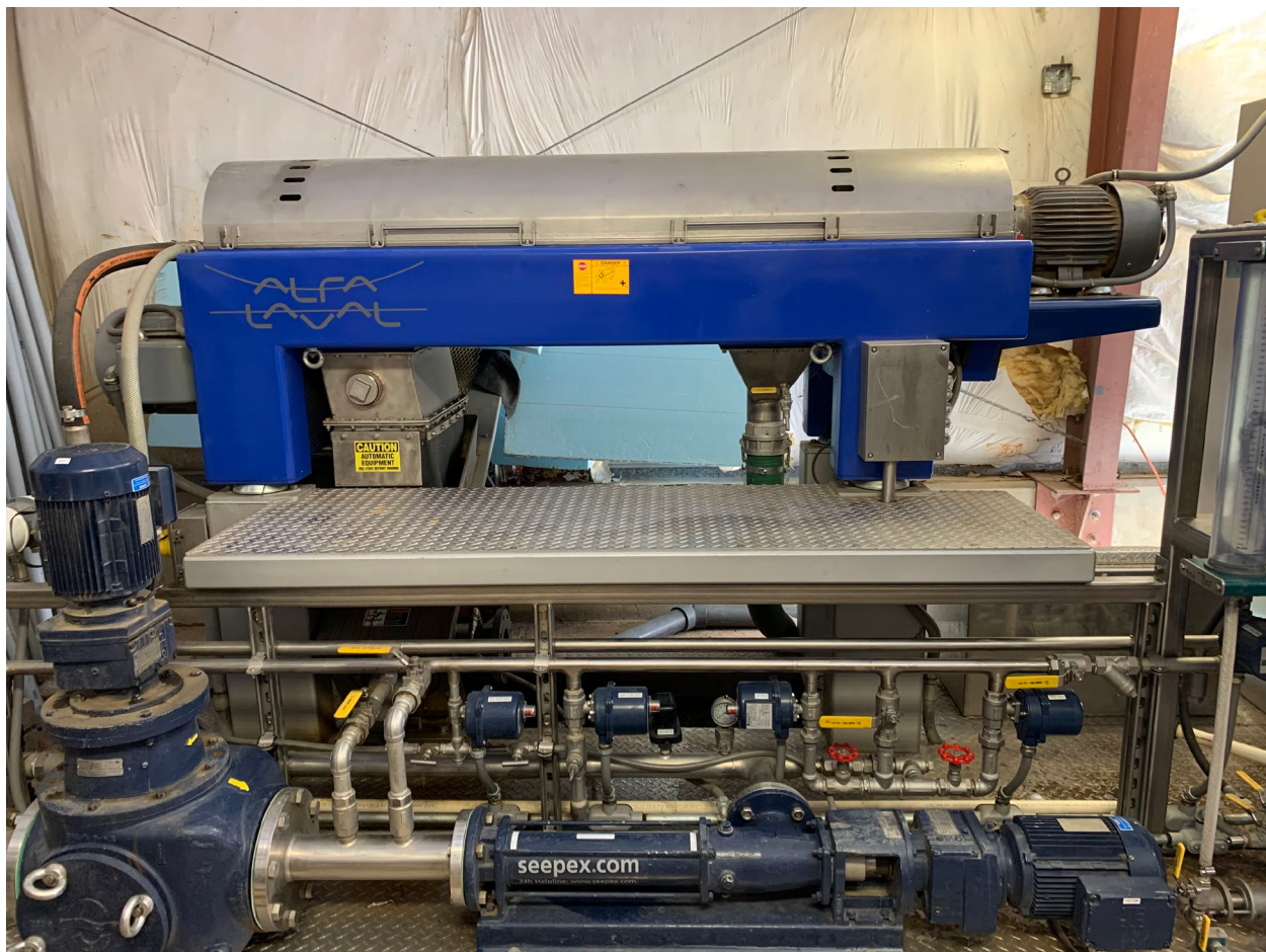
A view of the Alfa Laval centrifuge within the dewatering building. (IMG_0221). (10:43 AM:01/18/2024) Photographed by D. Esparza
