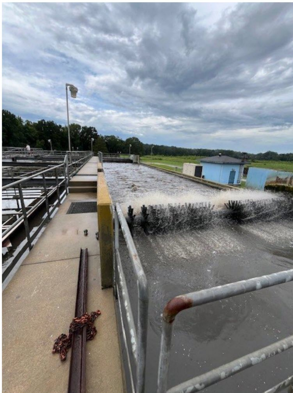
Racetrack with BOAT Clarifer
