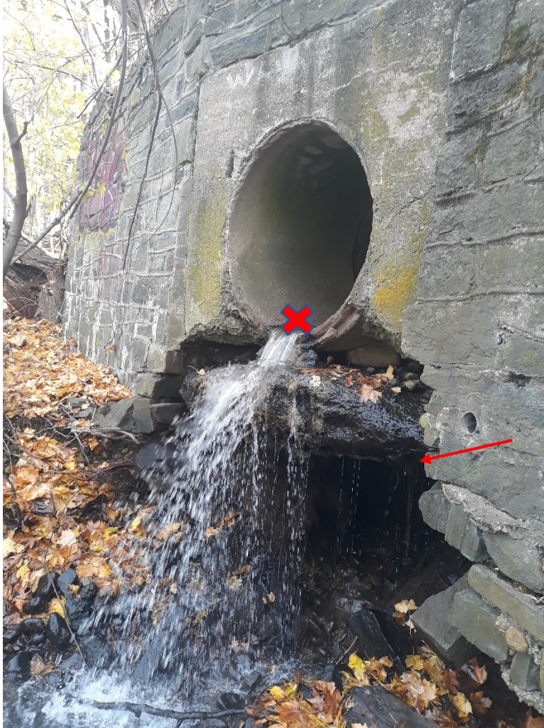
Ashley: Outfall located along Glenwood Avenue near the corner of Ashley Street. Note the discharge flowing under and behind the mouth of the outfall (red arrow), due to cracks in the piping joint and degradation of the reinforcement blocks. Sample point is indicated by a red “x”.
