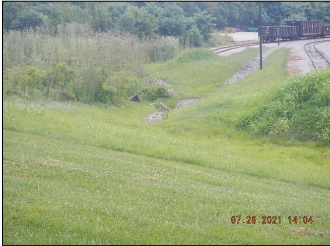
Photo 1: Inlet to Outfall 004.
