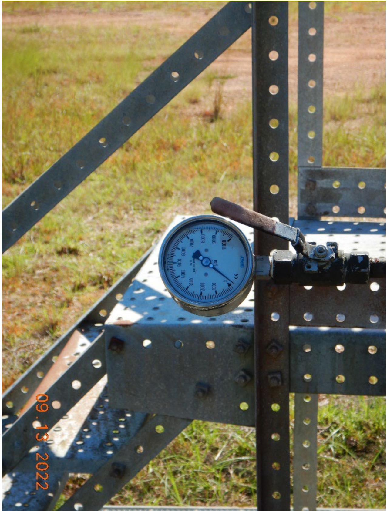
Photograph 4: Looking east, closeup view of internal pressure gauge reading 0 psi.
