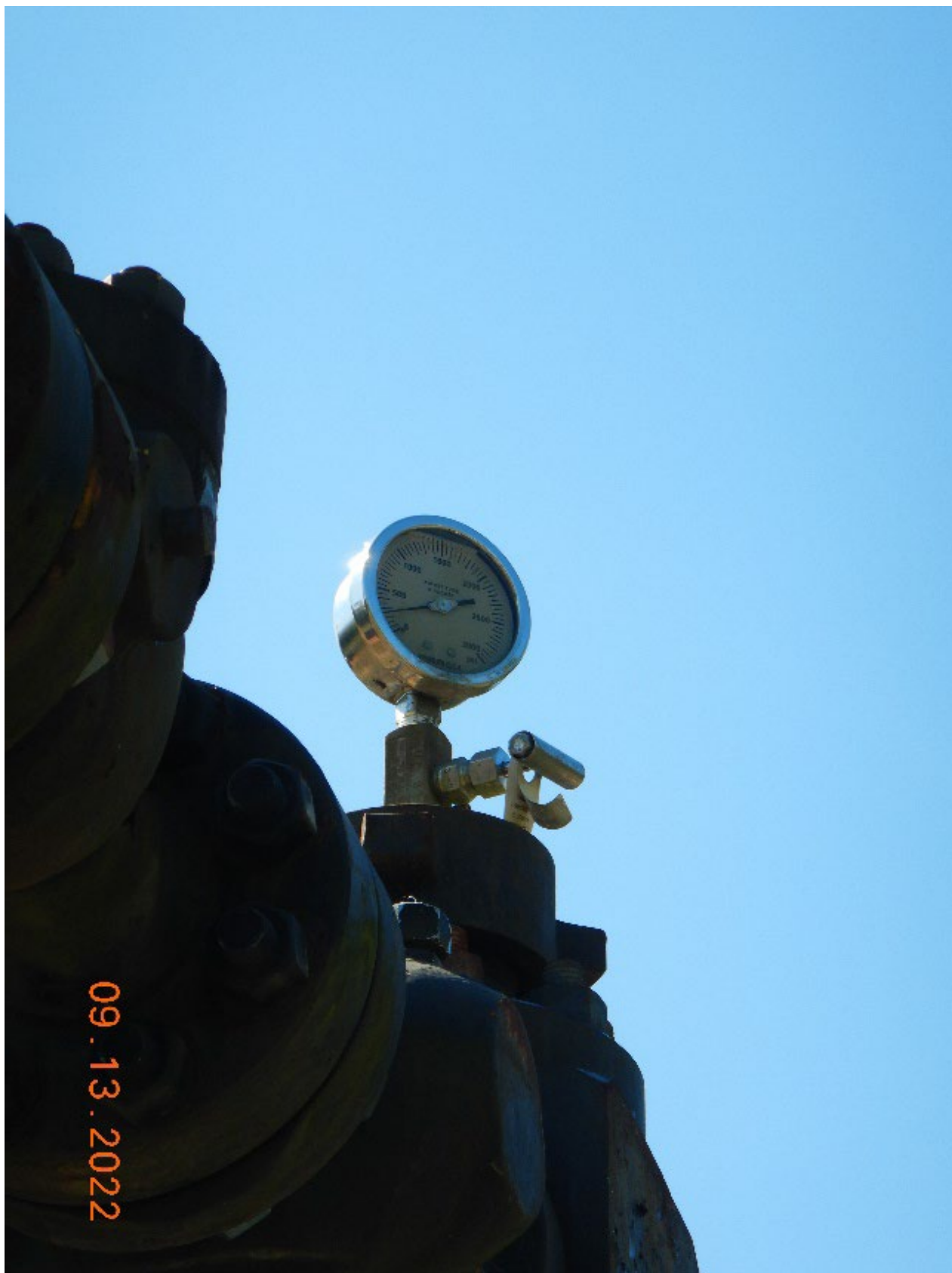
Photograph 5: Looking southeast, closeup view of internal pressure gauge reading 250 psi.
