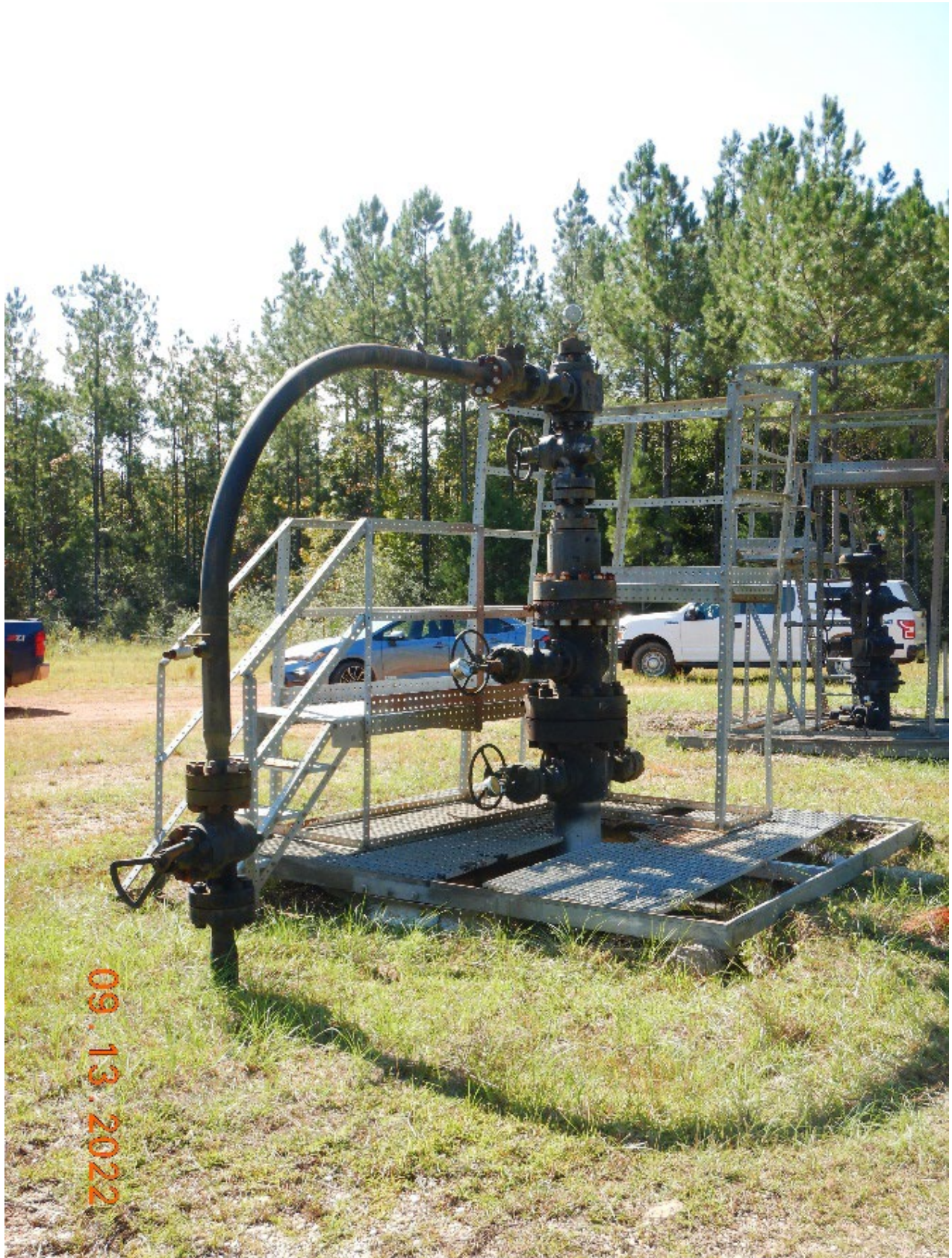
Photograph 2: Looking east, site overview, including well head, pressure gauges, valves, and access stairs.
