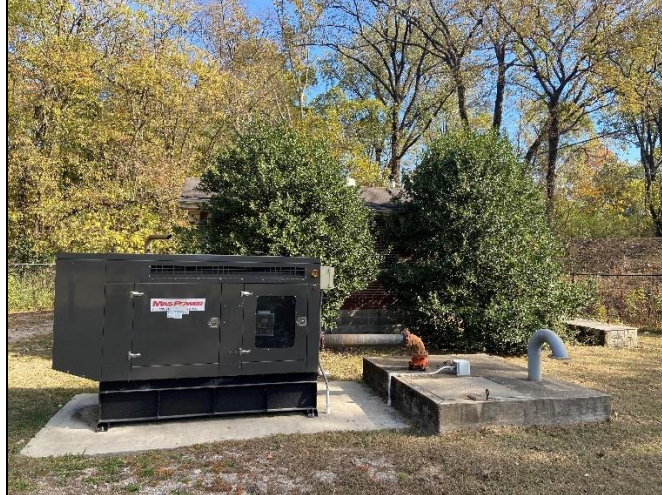
Photo 4: Red Farmer Way pump station.
