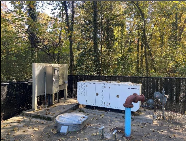
Photo 3: Chapel #2 pump station.
