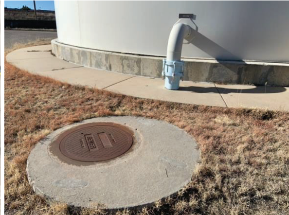
Effluent Tank Inlet (manhole)
