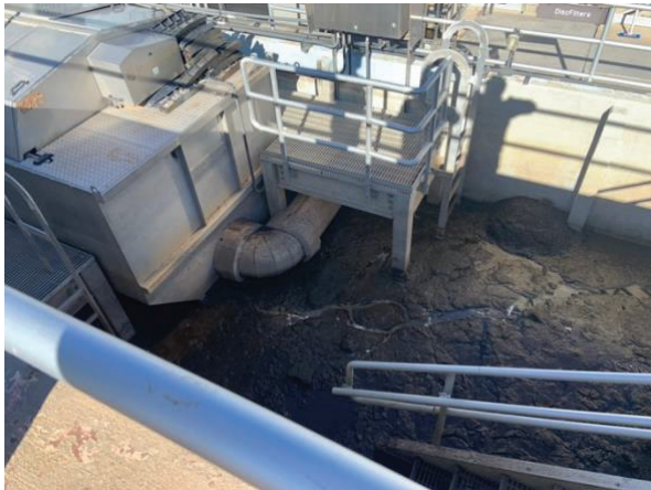
Photo 3: Sludge spilled from plant sump to UV enclosure
