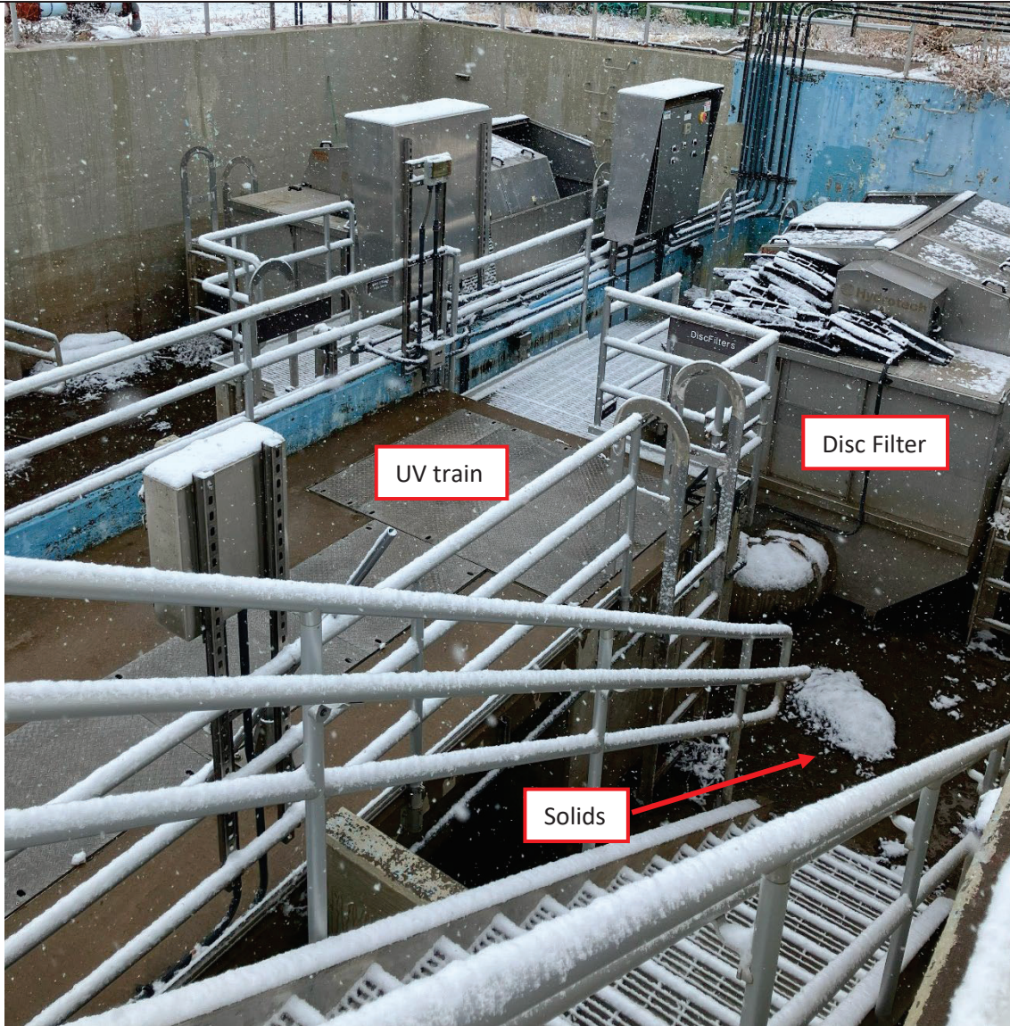
Solids in the UV channel and disk filter housing during the overflow event.
