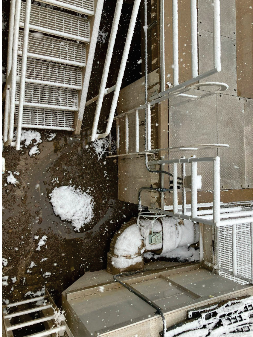
Solids in the UV channel and disc filter housing during the overflow event.
