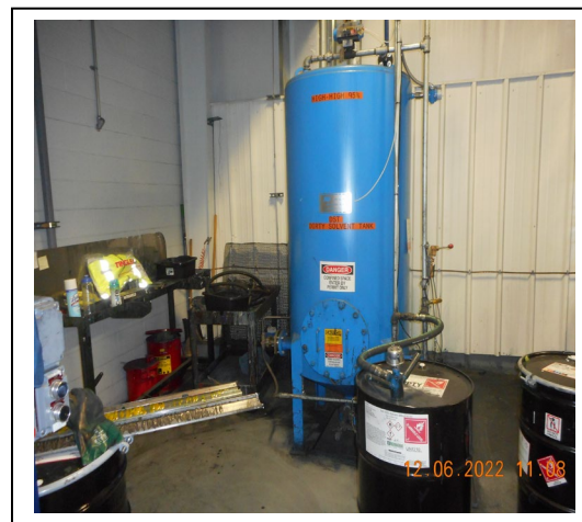
Photo #4 - 150-gallon spent solvent tank.
