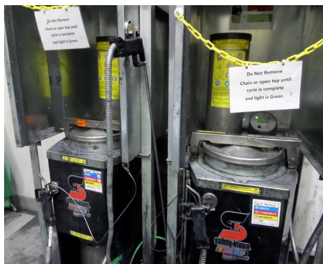
Slurry Building Distillation Area. The inspector observed two distillation units to recover spent acetone. Emissions are vented outdoors. Photograph 10 taken at 11:17 a.m.
