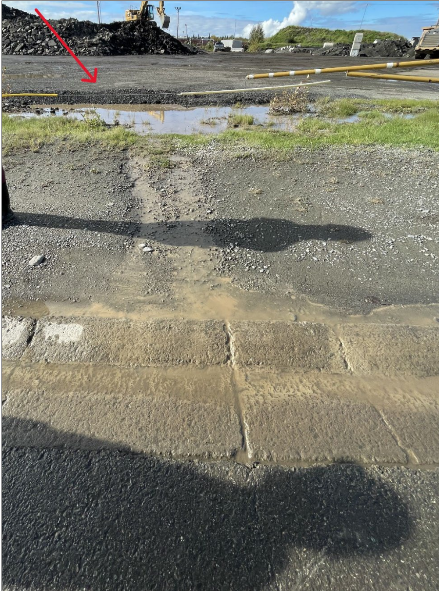
Picture 21: Discharge from RAP Processing Area
