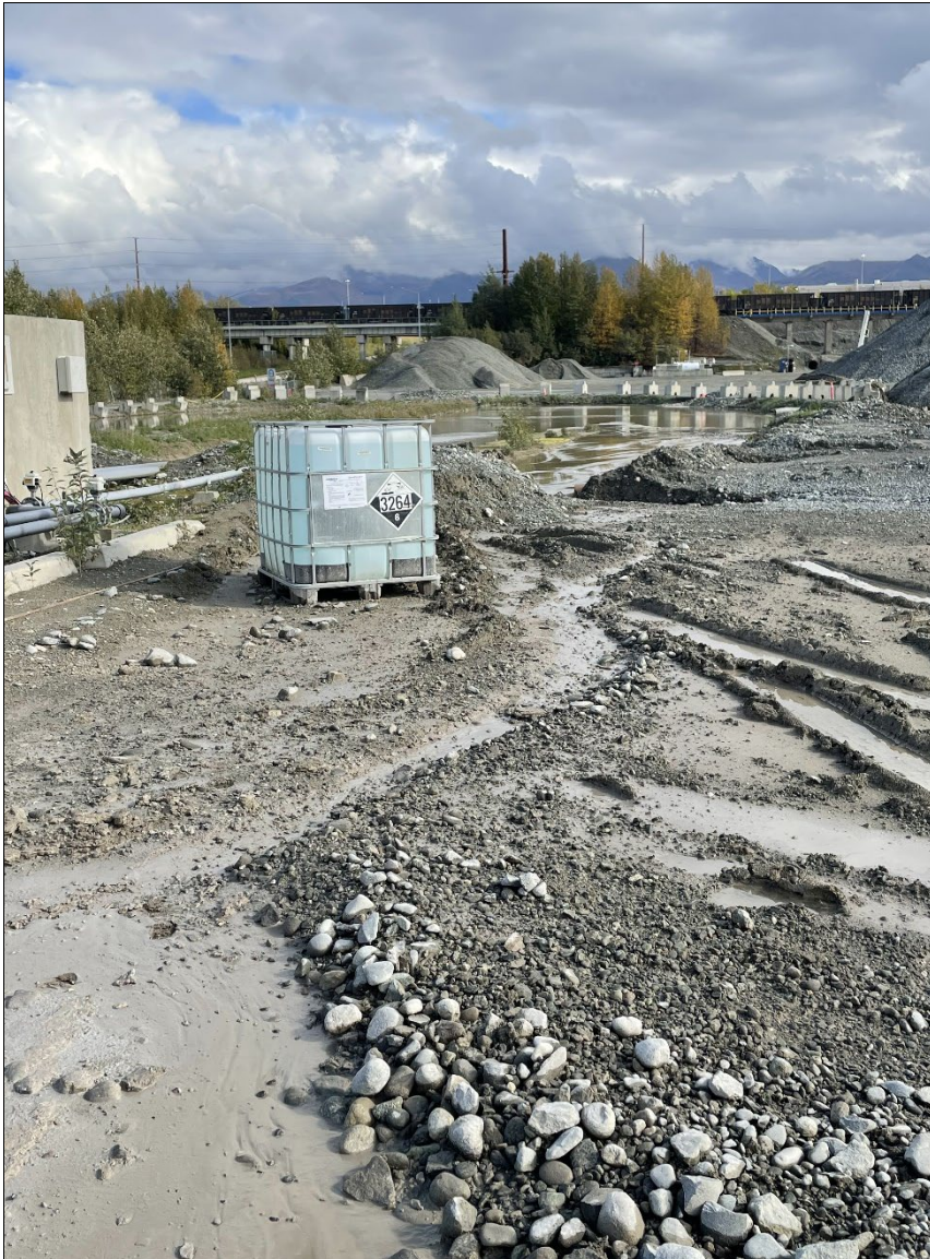
Picture 13: Material Stored in the Water Flow Path to Pond
