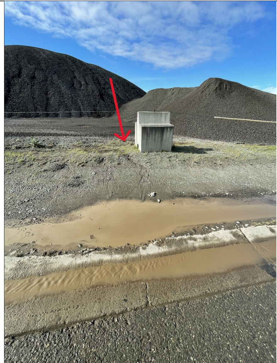
Picture 18: Discharge from RAP Processing Area
