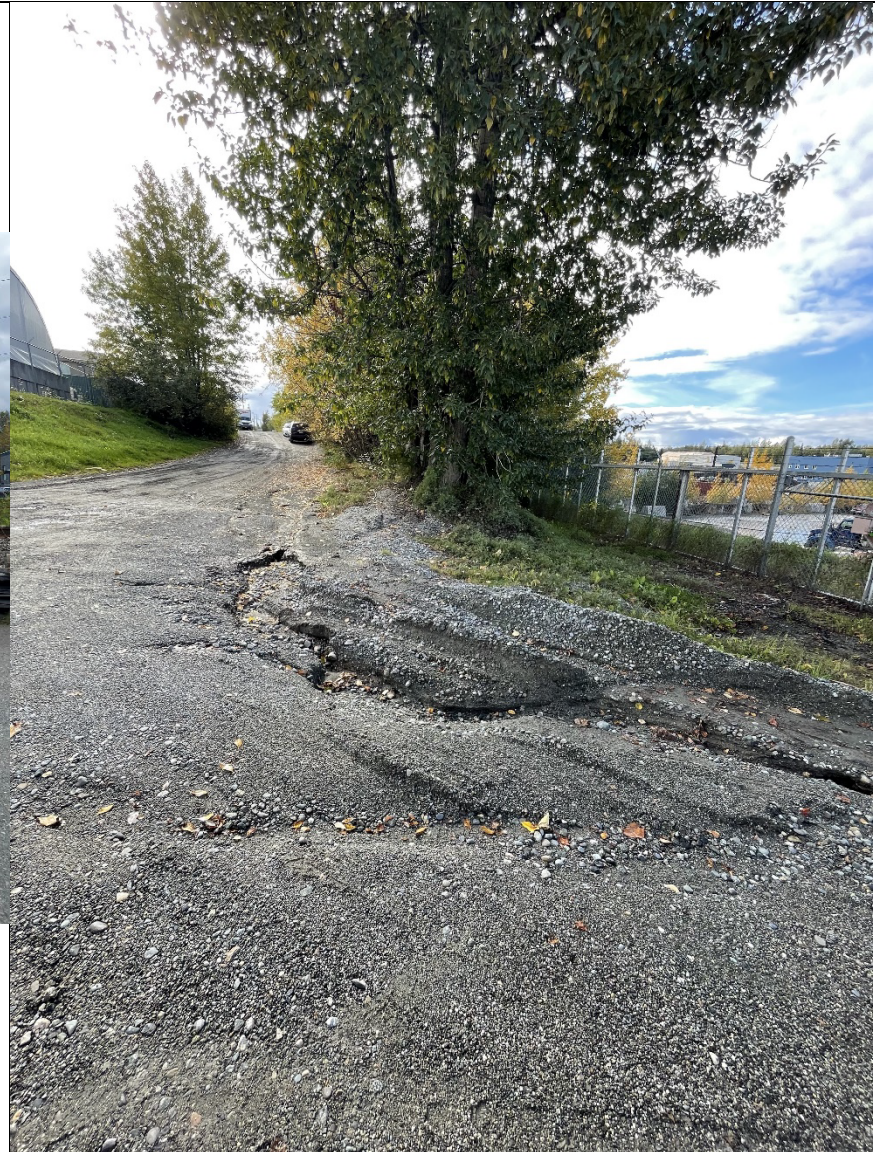
Picture 6: Evidence of Onsite Erosion
