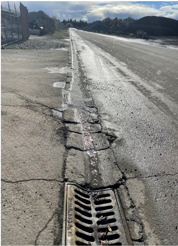
Figure 11: Discharge into Storm Drain at NE Corner of Lang Street & Gilman Parkway
