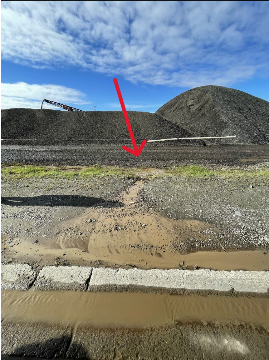
Picture 19: Discharge from RAP Processing Area
