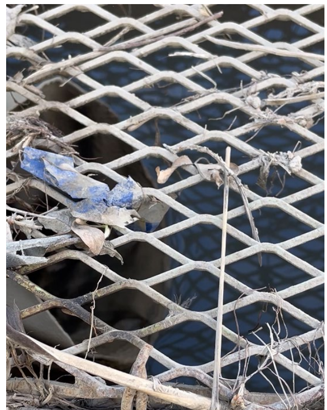
Figure 8: Overflow Pipe Discharging
