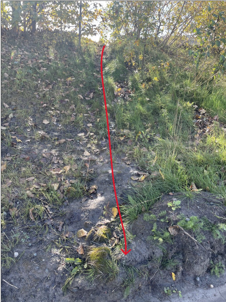
Picture 33: Sediment and Sediment Path from Discharge along Northern Facility Road
