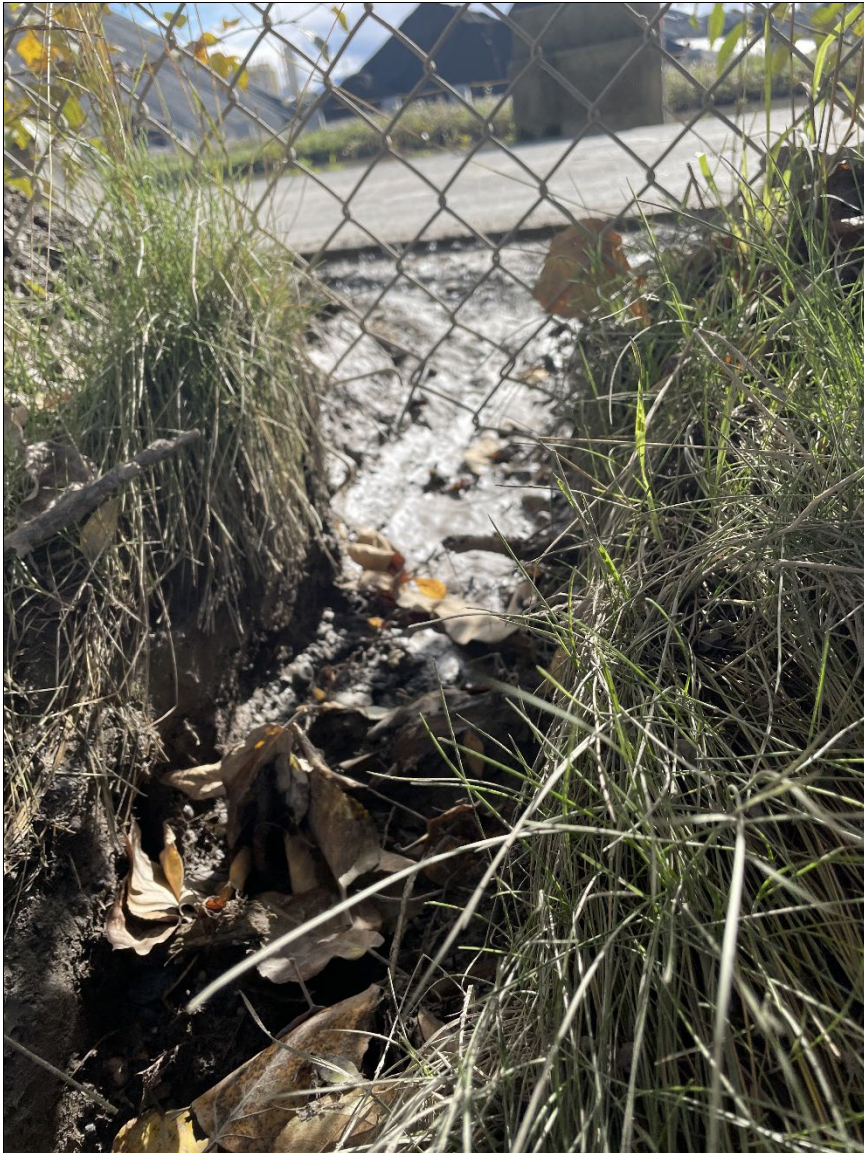
Picture 29: Discharge along Northern Facility Road
