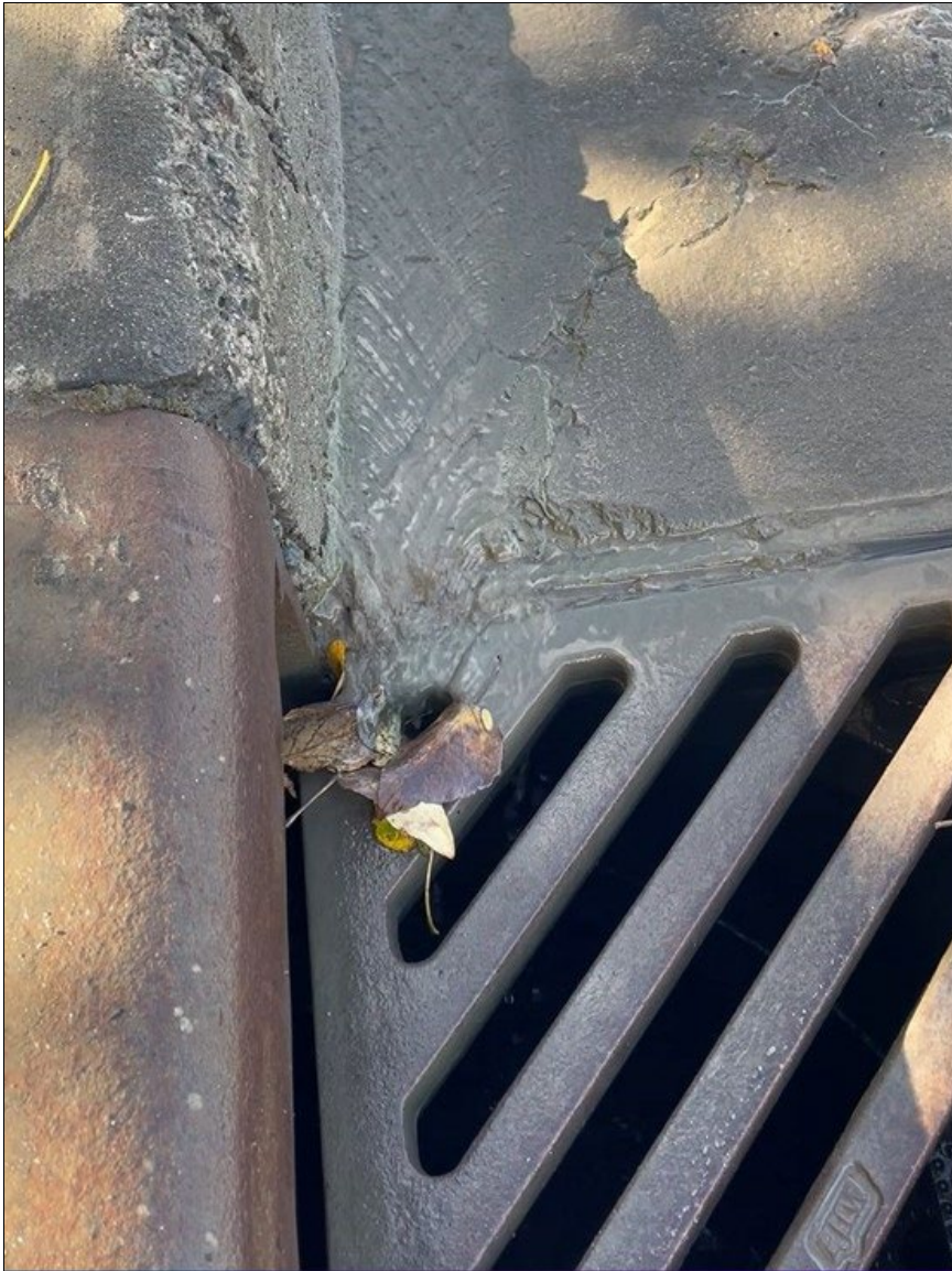
Picture 35: Discharge from AS&G into Storm Drain in Gilman Pkwy.
