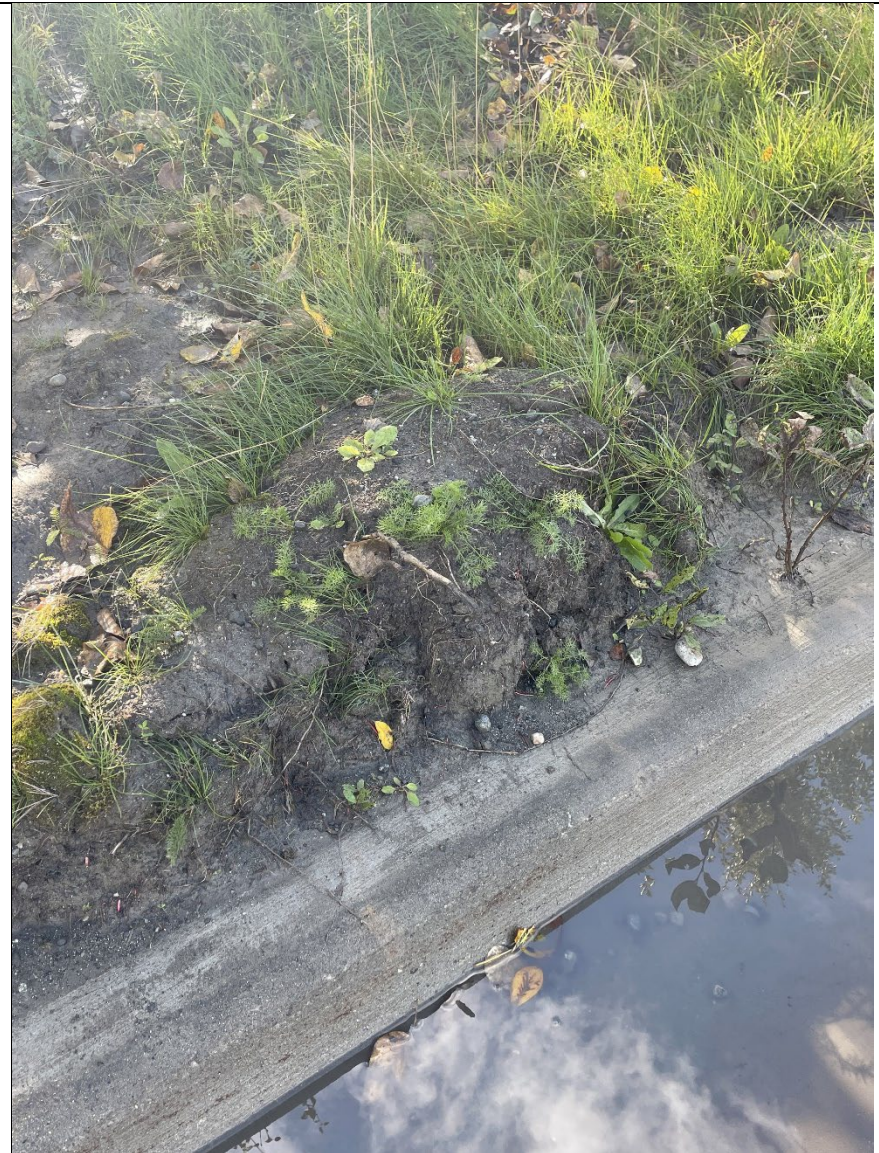
Picture 32: Buildup of Sediment from Discharge along Northern Facility Road
