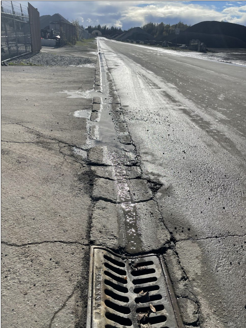
Picture 27: Discharge at NE Corner of Lang St. and Gilman Pkwy.
