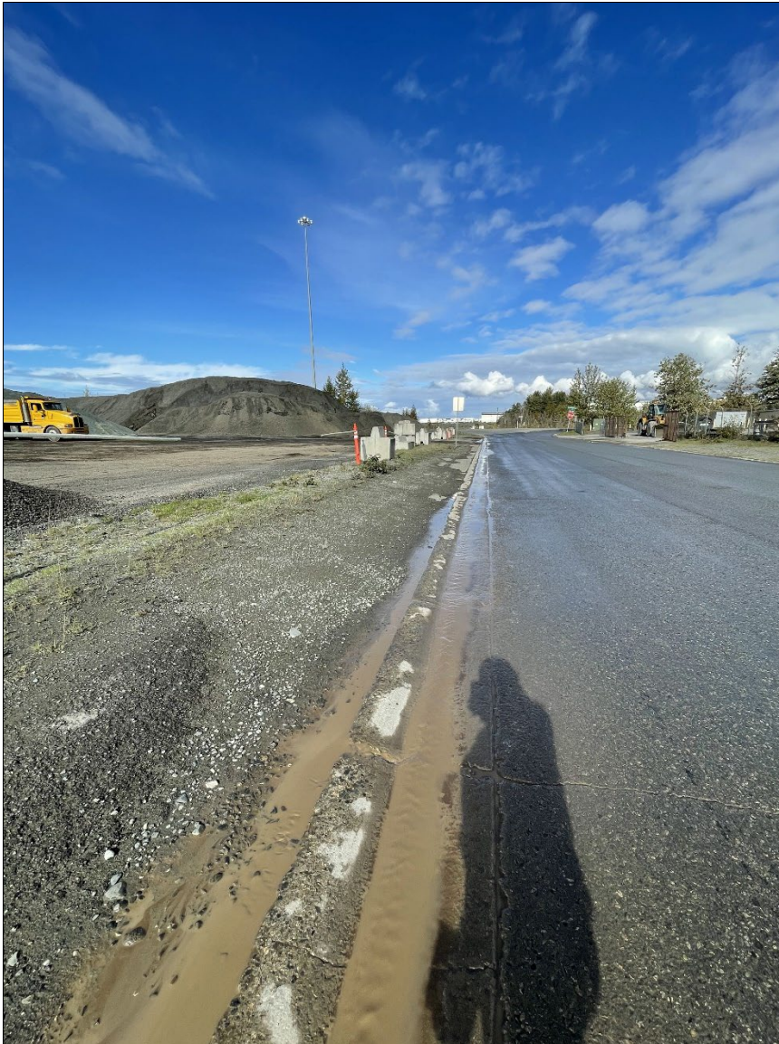
Picture 17: Discharge from RAP Processing Area
