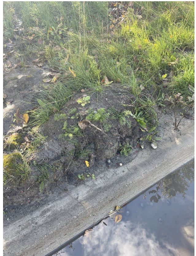
Figure 6: Sediment Deposit and Curb
