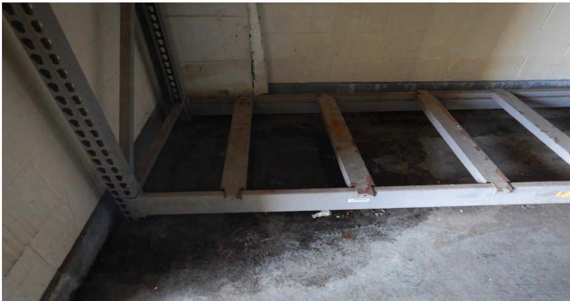
404 – Liquid on the ground inside building 1582
