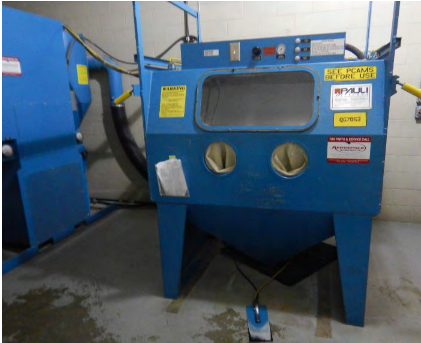
466 – Building 282 Sand blast unit
