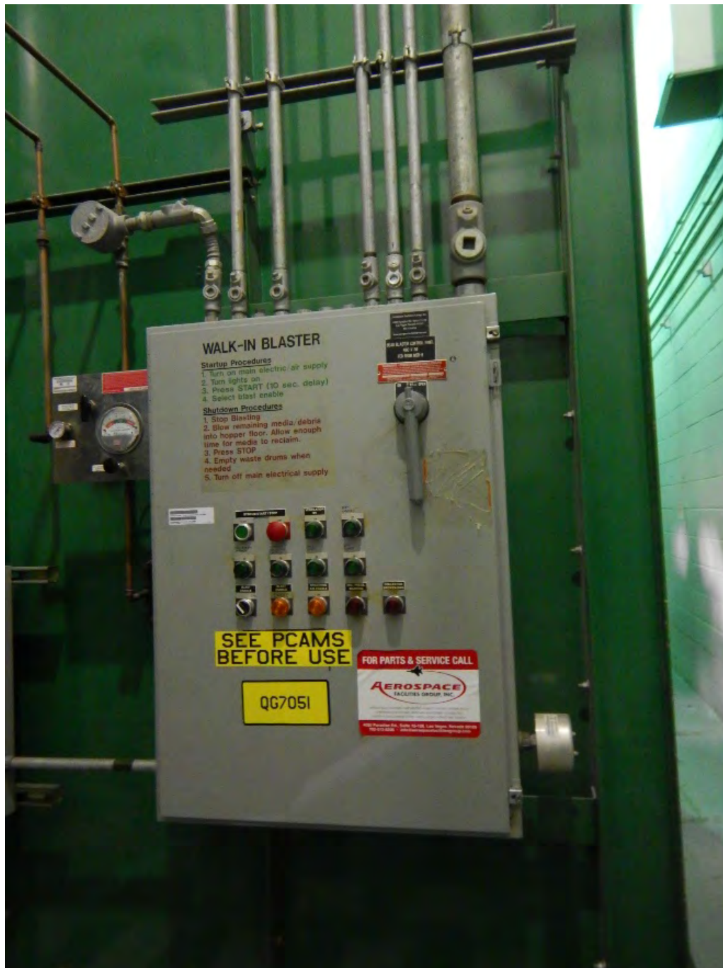
473 – Operation controls for walk in blaster building 282
