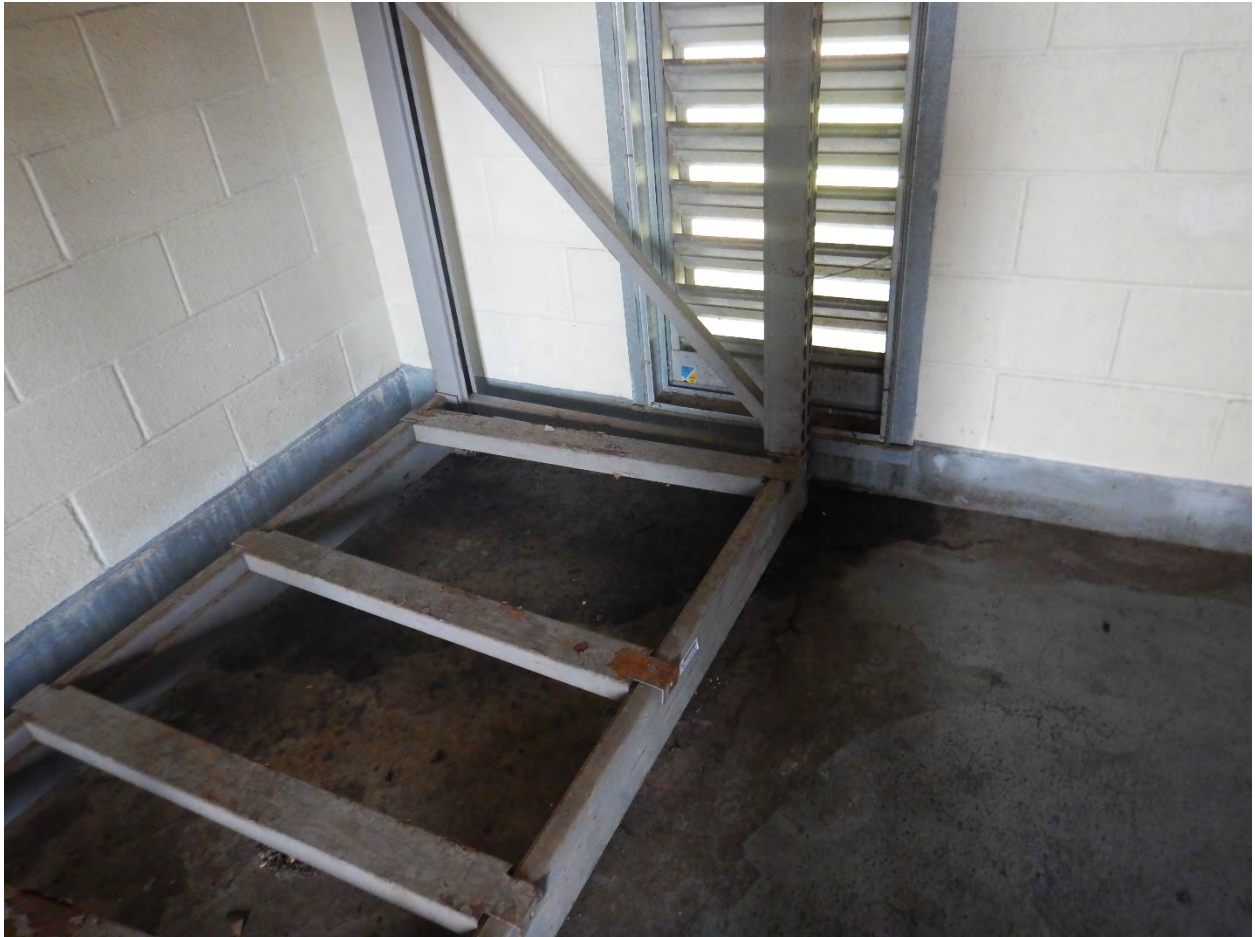
405 - Liquid on the ground inside building 1582
