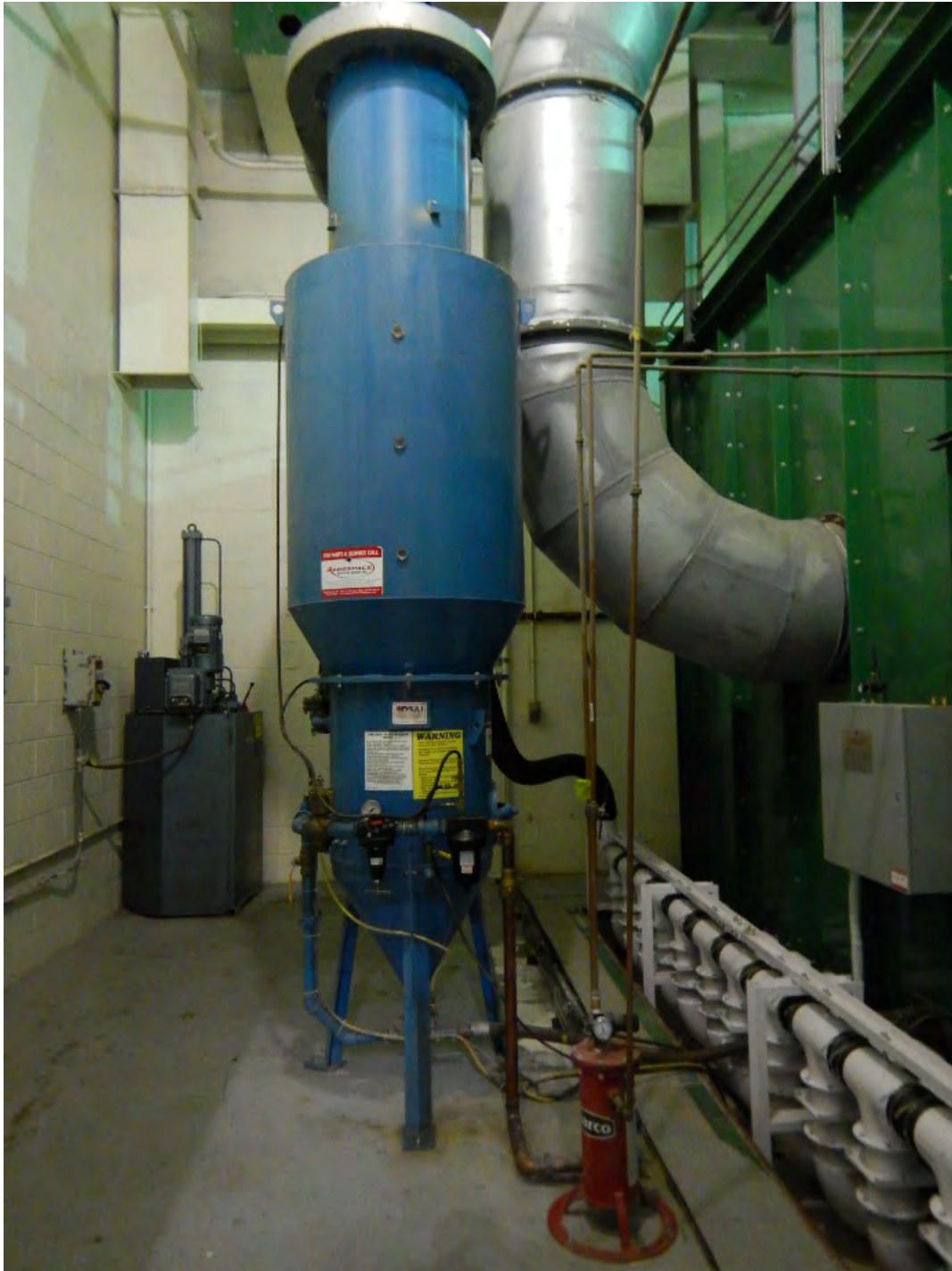
475 – Walk in blast unit building 282
