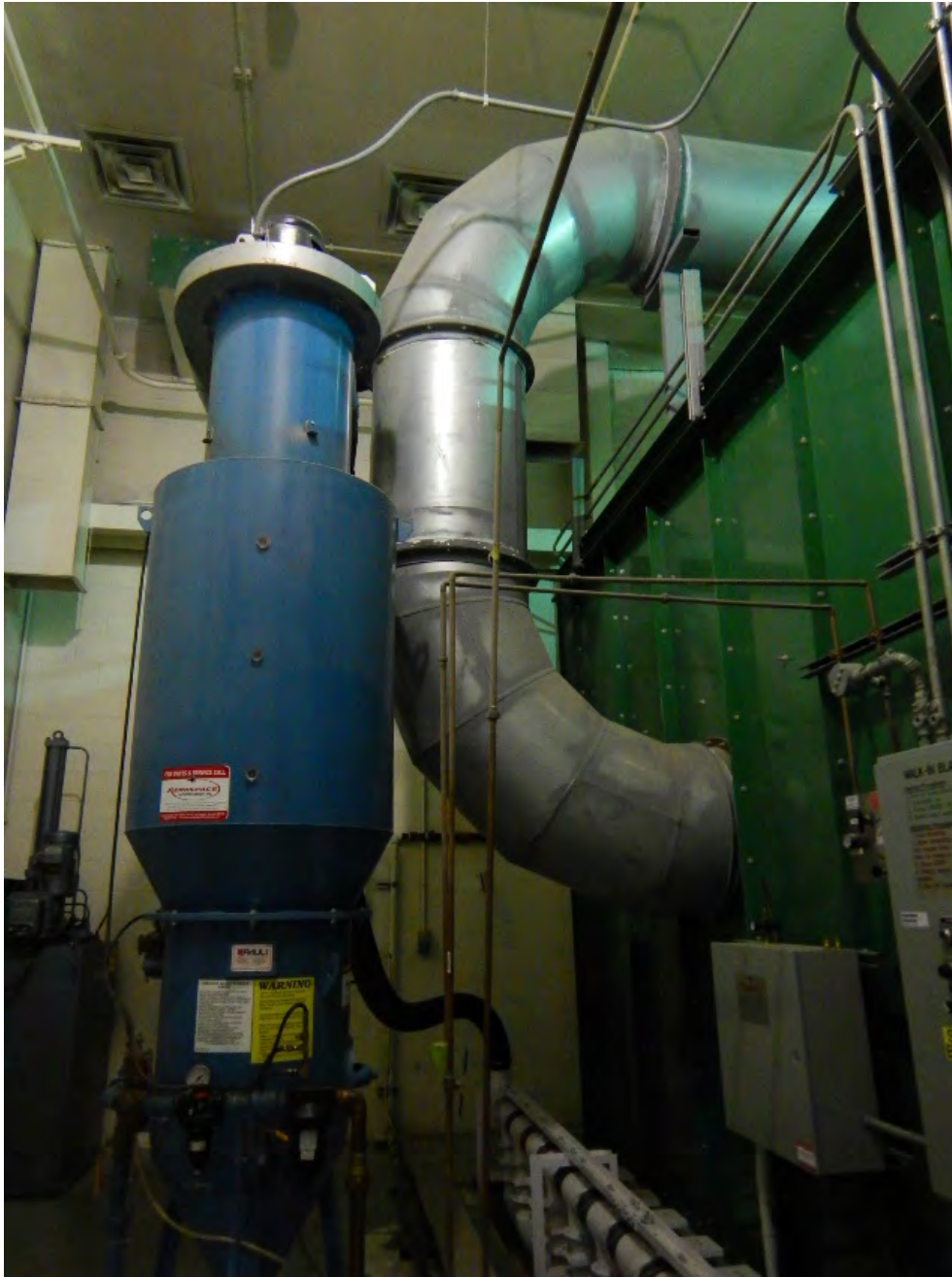
476 – Walk in blast unit building 282
