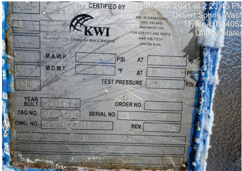
Photograph 8 – JT Skid related
