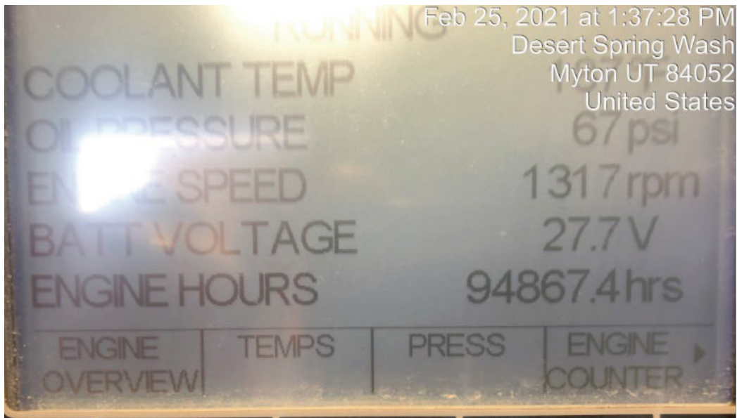
Photograph 2b – RB#3 Runtime
