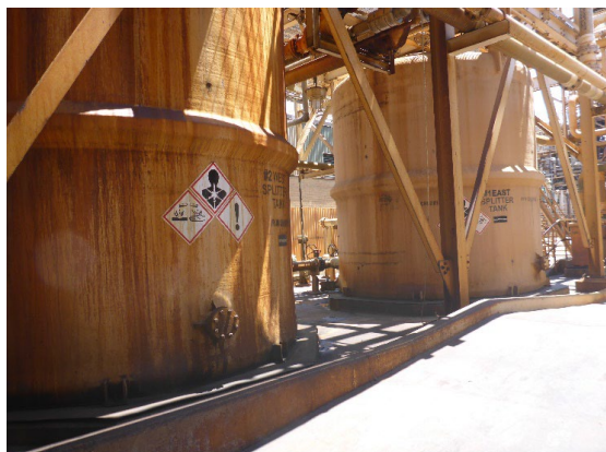
Photo 5: Splitter Feed Tanks.
