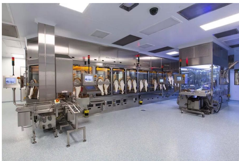
Figure 4.3: Isolator in cleanroom (source: Optima).
