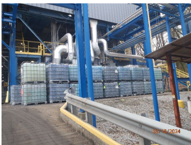
Picture 13 – Copper Oxide Plant totes to be reworked
