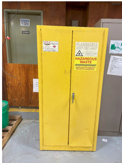
Picture 45 – Tech Center Pilot Plant flammable cabinet SAA
