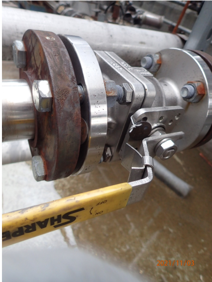
Photo 13: The ancillary equipment was marked/ tagged as required by Subpart BB. The tags however were illegible due to dirt/ dust.
