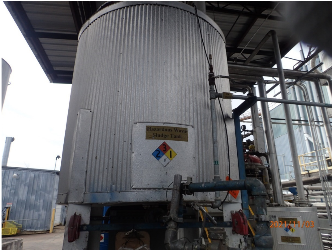
Photo 6: 750-gallon storage tank for hazardous waste still bottoms labeled “Hazardous Waste Tank Sludge” and marked with an indication of hazard.
