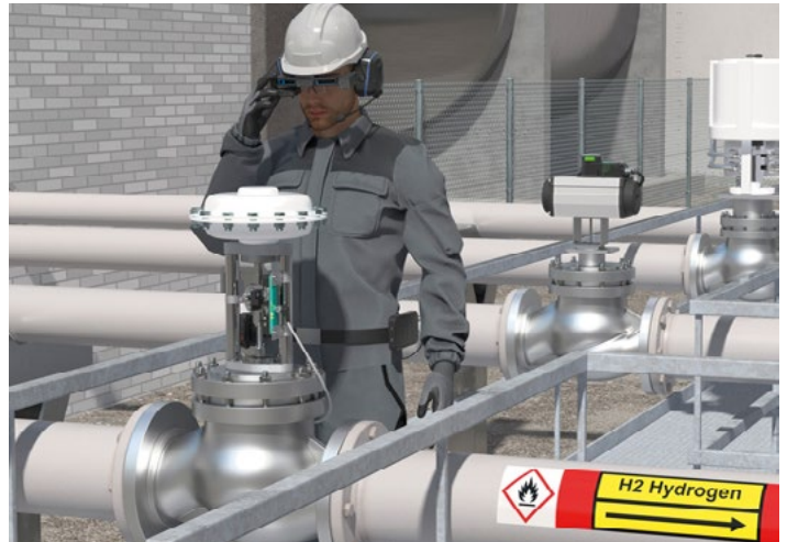
The PMI inductive position measuring system reliably detects the valve position on the hydrogen pipelines, as well.
