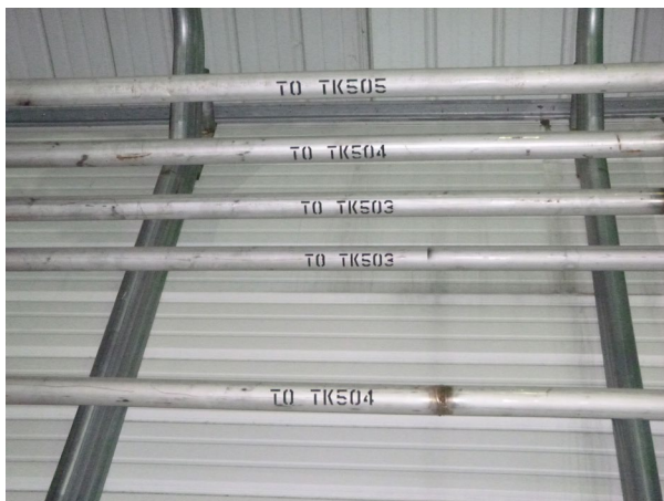
Photograph 35: Hazardous Waste CAA Tank ancillary equipment.
