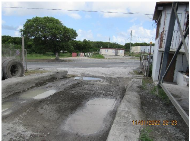
IMG 780 -Close-up of the ready-mixed concrete loading bay, inclined down towards the public road.
