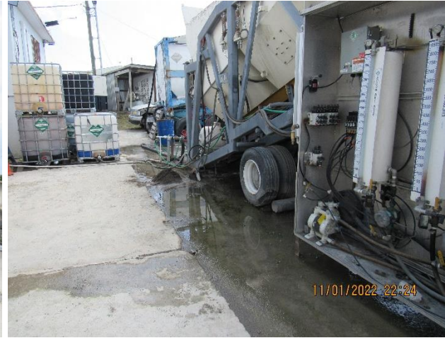
IMG 783 -Close-up of accumulated water beneath the batch plant, and point where dry-weather flow observed began.
