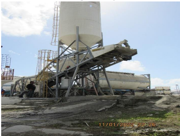
IMG 786 -View of ready-mixed concrete loading bay, the wider ready-mixed manufacturing plant, situated adjacent to the Admin Office.
