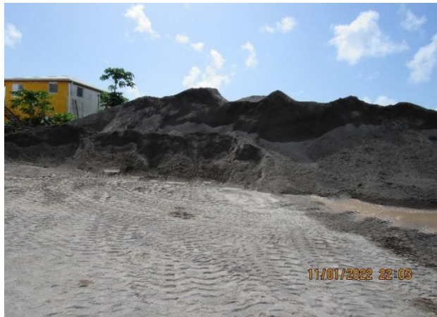
IMG 760 -Storage cell with sand situated about mid-way along the eastern border of the Facility. Cell is exposed to rain and stormwater runoff flow.
