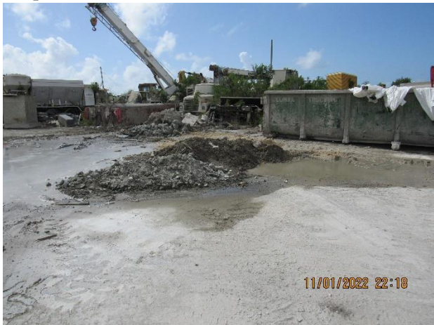
IMG 773 -Edge of the pond where spent concrete to a berm. The berm ineffective because a dry-weather flow drained from the pond. and out of the Facility. wastewater).
