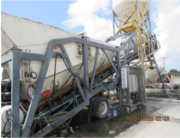
IMG 785 -Accumulation of water beneath ready-mix Ed concrete batch plant related to operations of the system. Source of a dry-weather flow observed.
