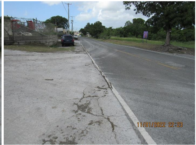
IMG 782 -Evidence of track-out of pollutants from Facility and into the public road. Path of stormwater runoff leaving the Facility from upper entrance/exit.
