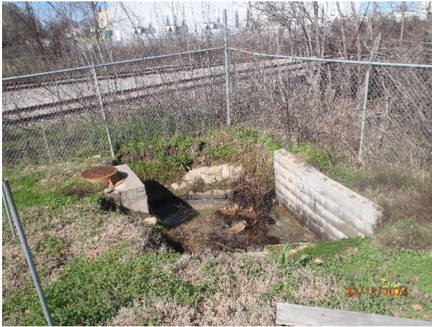
Picture 13 – Sump Collection Basin
