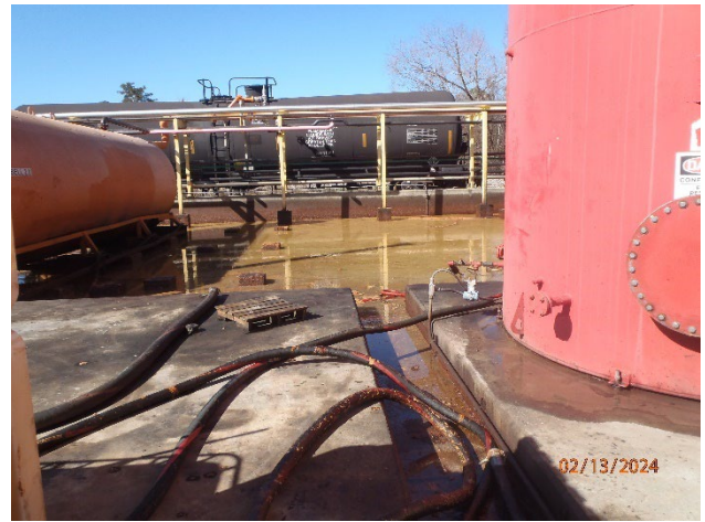
Picture 10 – Day Tank Farm containment flooding
