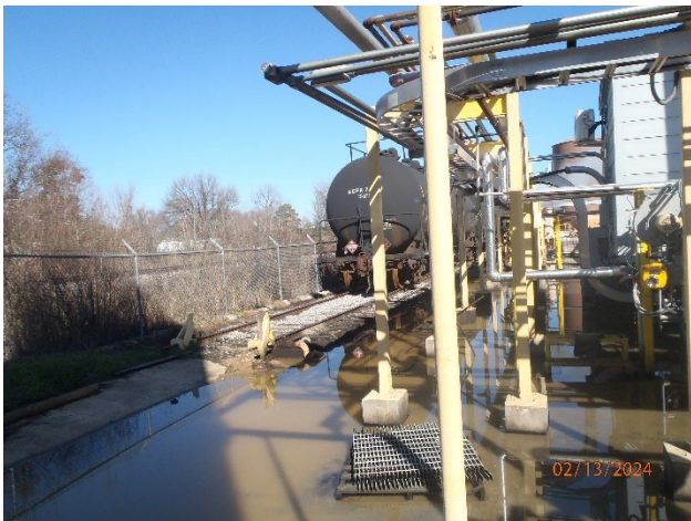
Picture 9 – Flooding along the railway
