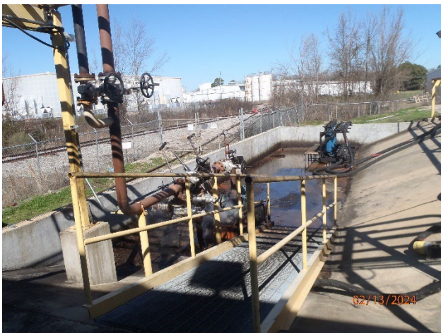
Picture 21 – Corn Oil unloading area and secondary containment
