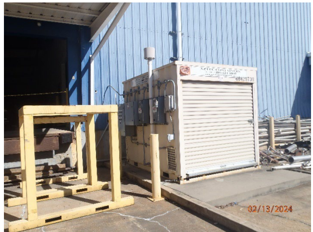
Picture 24 – Vapor Intrusion Building and Alarms
