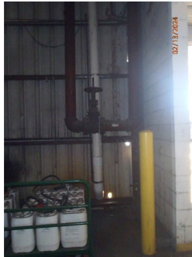
Picture 28 – Vapor Intrusion piping
