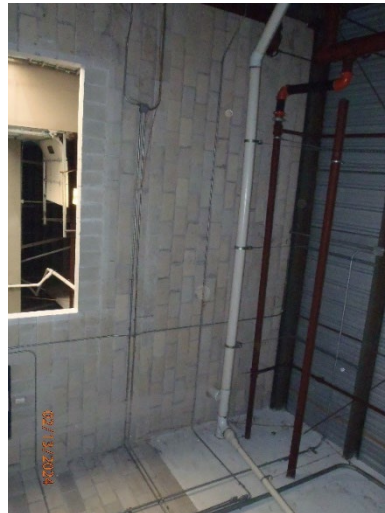
Picture 29 – Vapor Intrusion piping
