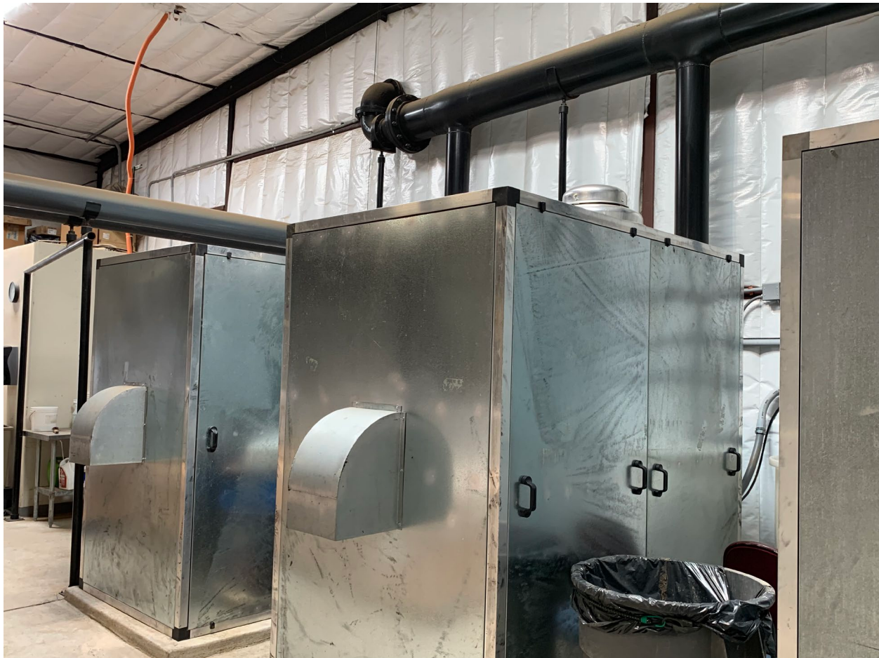
View of two (2) of the three (3) WWTP blowers. Note: one (1) blower required extensive repair after catching fire. (IMG0147). September 13, 2022. Photographed by D. Esparza
